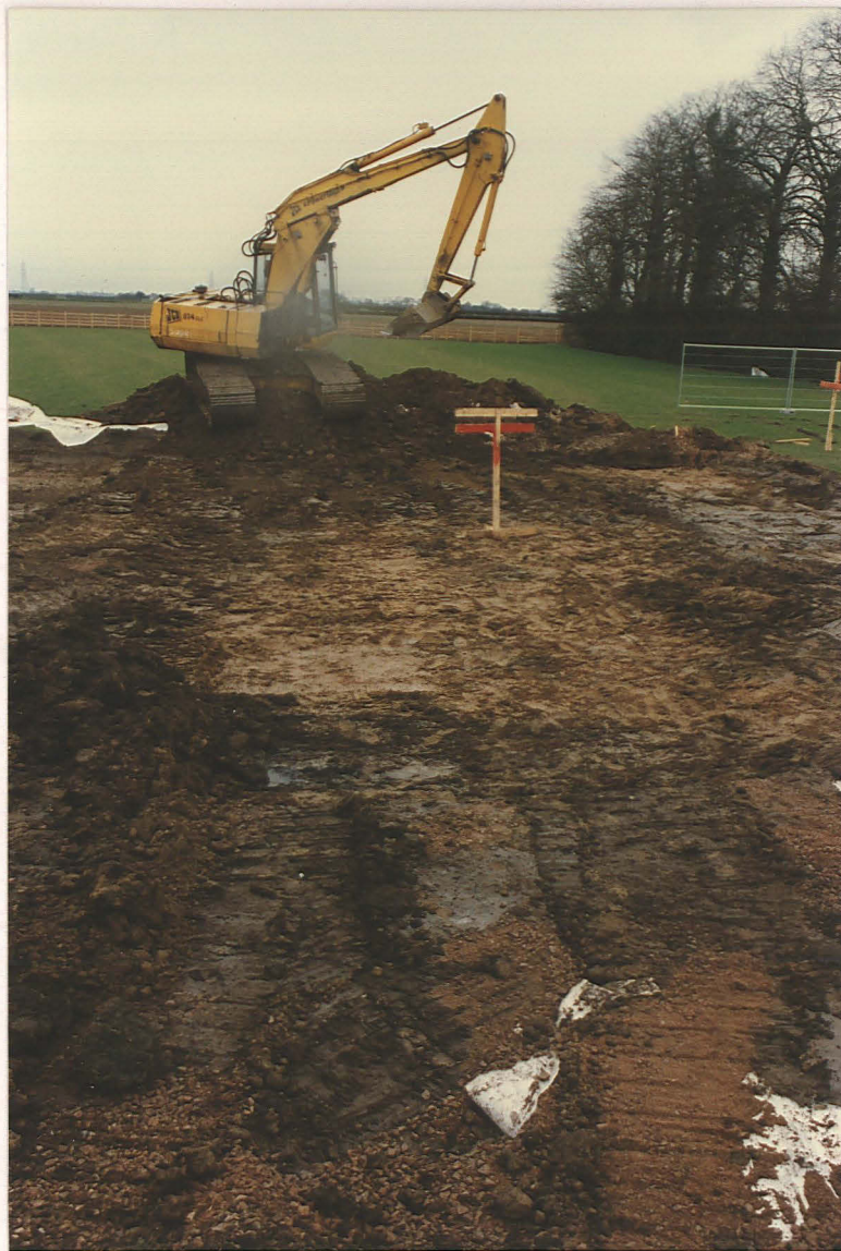
Pl. 5 Stone chippings (foreground) removed to lower ground level a further 3-400mm. Looking NE.
