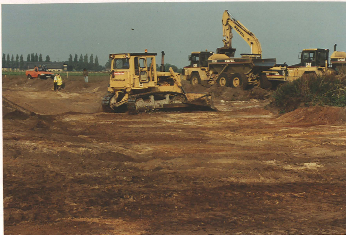
Pl. 22 Topsoil stripping at the southern part of the area, in the vicinity of concrete demolition rubble (far right) and a concrete wall foundation (in front of bulldozer). Looking NW.
