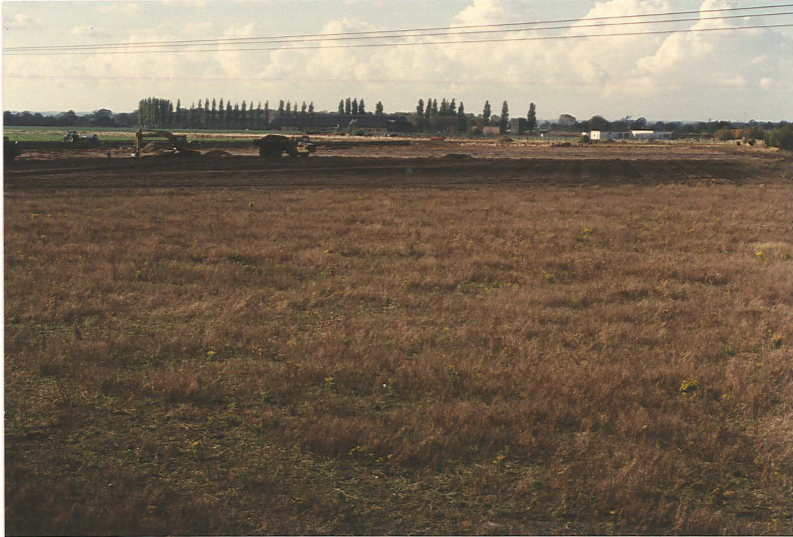
Frontispiece: Topsoil stripping in progress in Area 1b (looking NW towards golf course and RAF Woodhall premises. The existing quarry is to the right).
