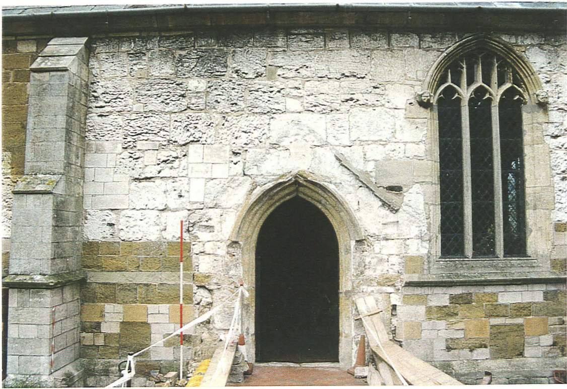
Plate 1: Area of Development. Showing entrance in medieval south nave wall and 'ghost' of 18th century porch
