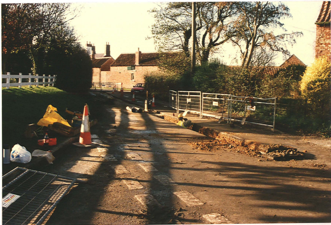
PI. 6 Trenching at 8 close to the junction of Louth Road and Chapel Lane (looking SW).
