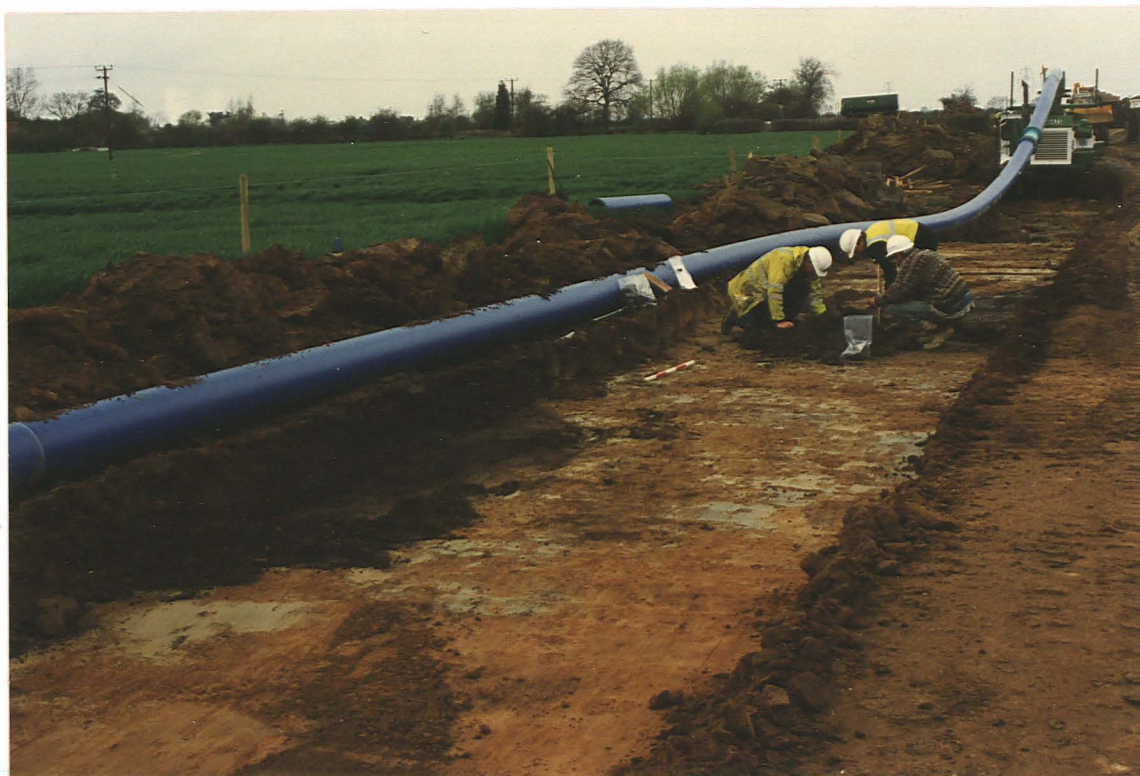
Pl. 16. Contractors helping to retrieve Iron Age pottery from ditch terminal 307 in advance of pipe-laying; ditch terminal 308 is visible as black soil (left foreground). Looking NW.
