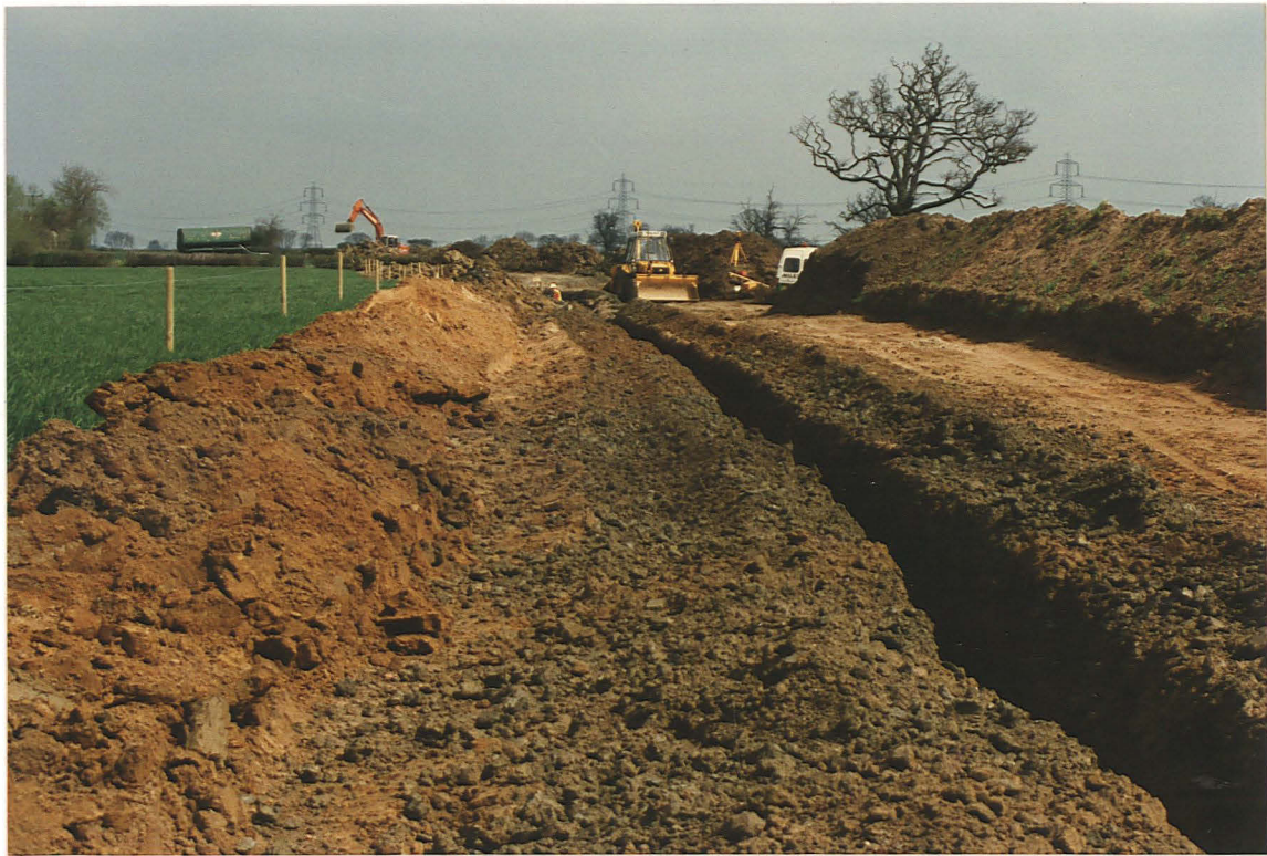
Pl. 19 The pipe trench was excavated across the Iron Age ditch terminals before detailed archaeological excavation began (looking north).
