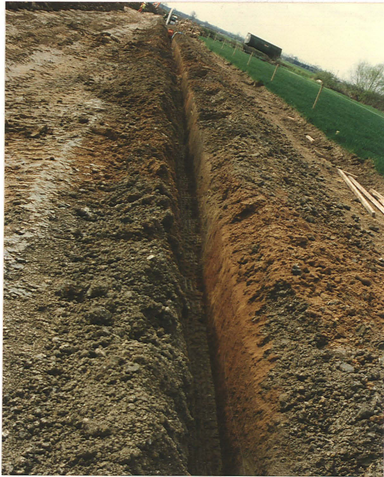
PI. 43 Mixed natural deposits of grey clay and sand in the faces of the pipe trench, Field 10 (looking south).
