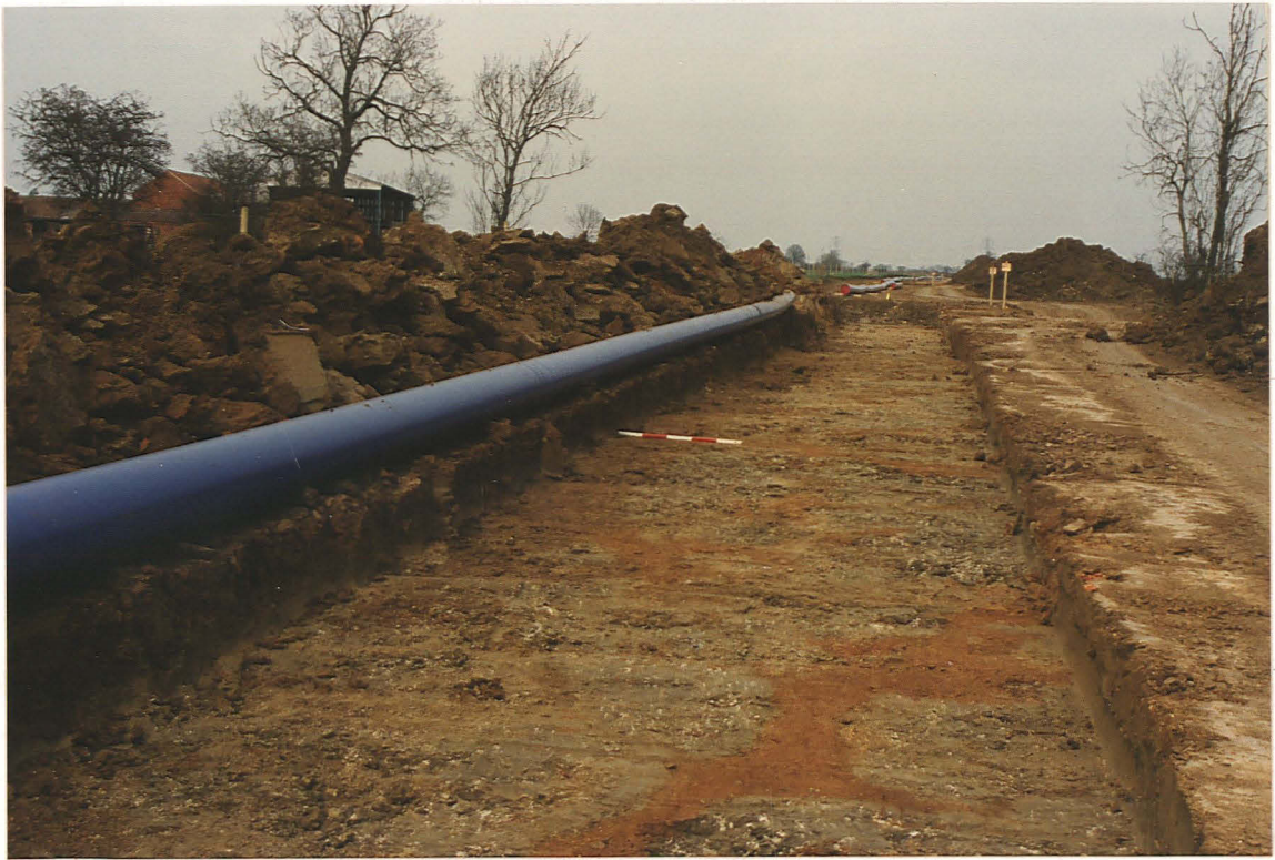
Pl. 50 Deeper aching of the easement SE of The Grange (Field 18) revealed the brown fill of a ditch (along edge beneath 1m scale; looking north).
