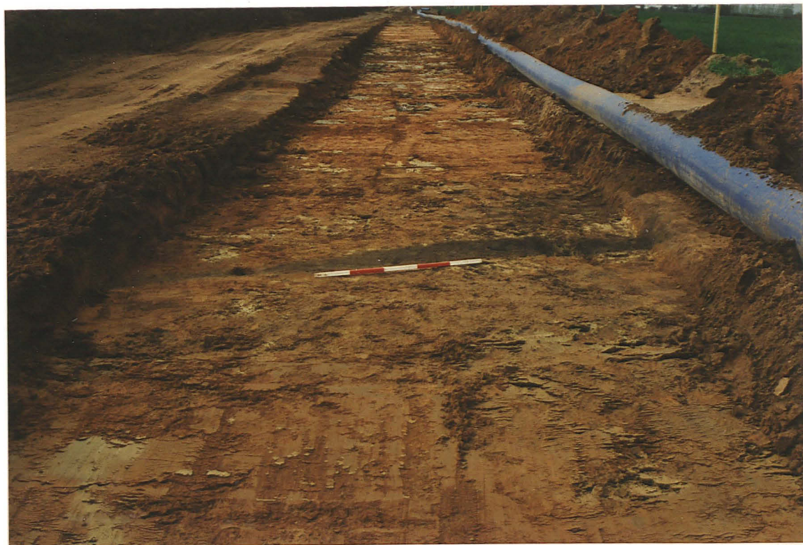
Pl. 12. Gully 136 visible only in the deeper machined strip. Part of Iron Age gully 101 is visible behind the pipe, centre right. Scale divisions 0.2m.
