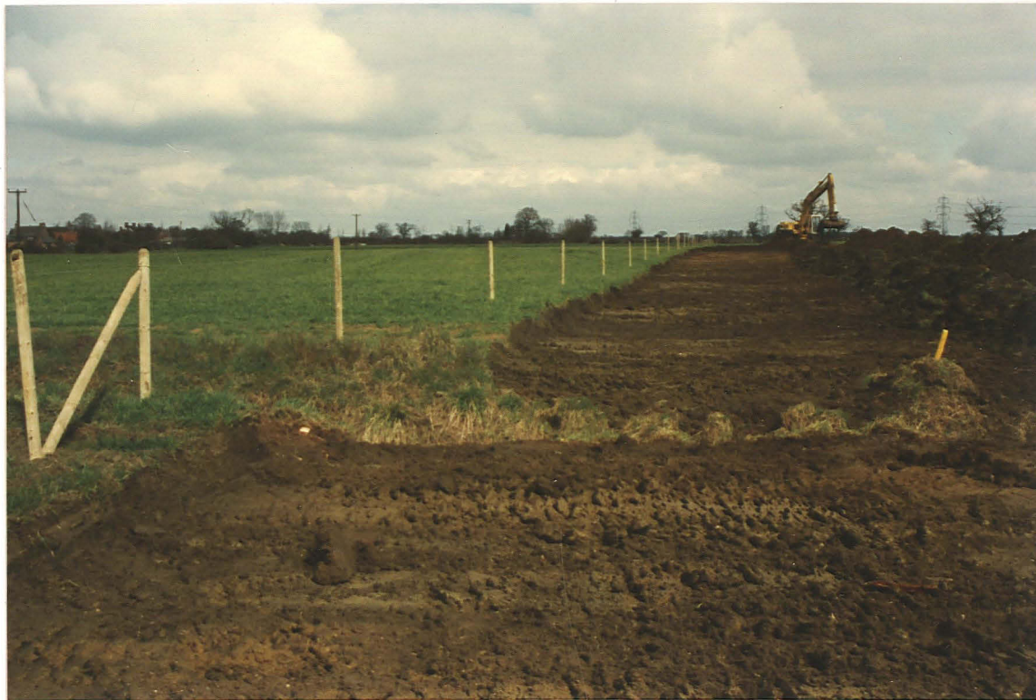
Pl. 15. During topsoil stripping in Field 12 a raised area of sandier soil was noted, coinciding with gullies 101 and 136 (looking N from Field 13 into Field 12; sandy soil beside machine).
