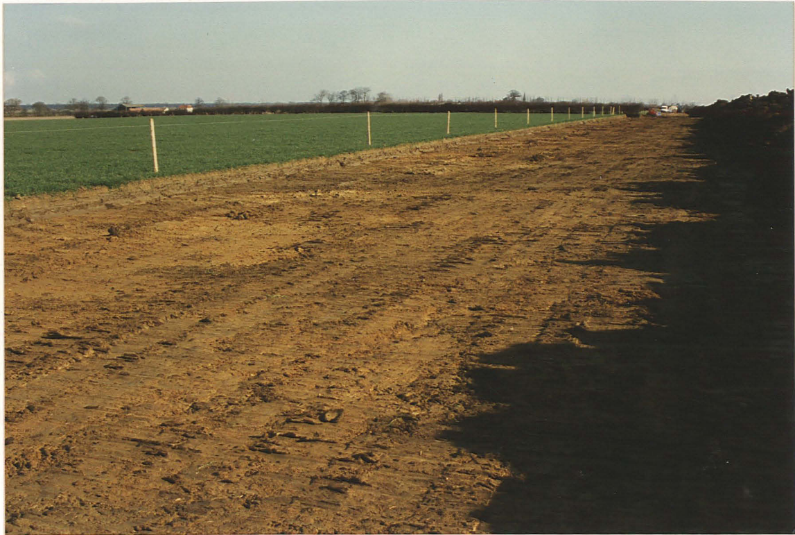
Pl. 76 Field 23 after topsoil stripping. Limestone rubble spread 23D is close to the nearest fence post (looking NW).
