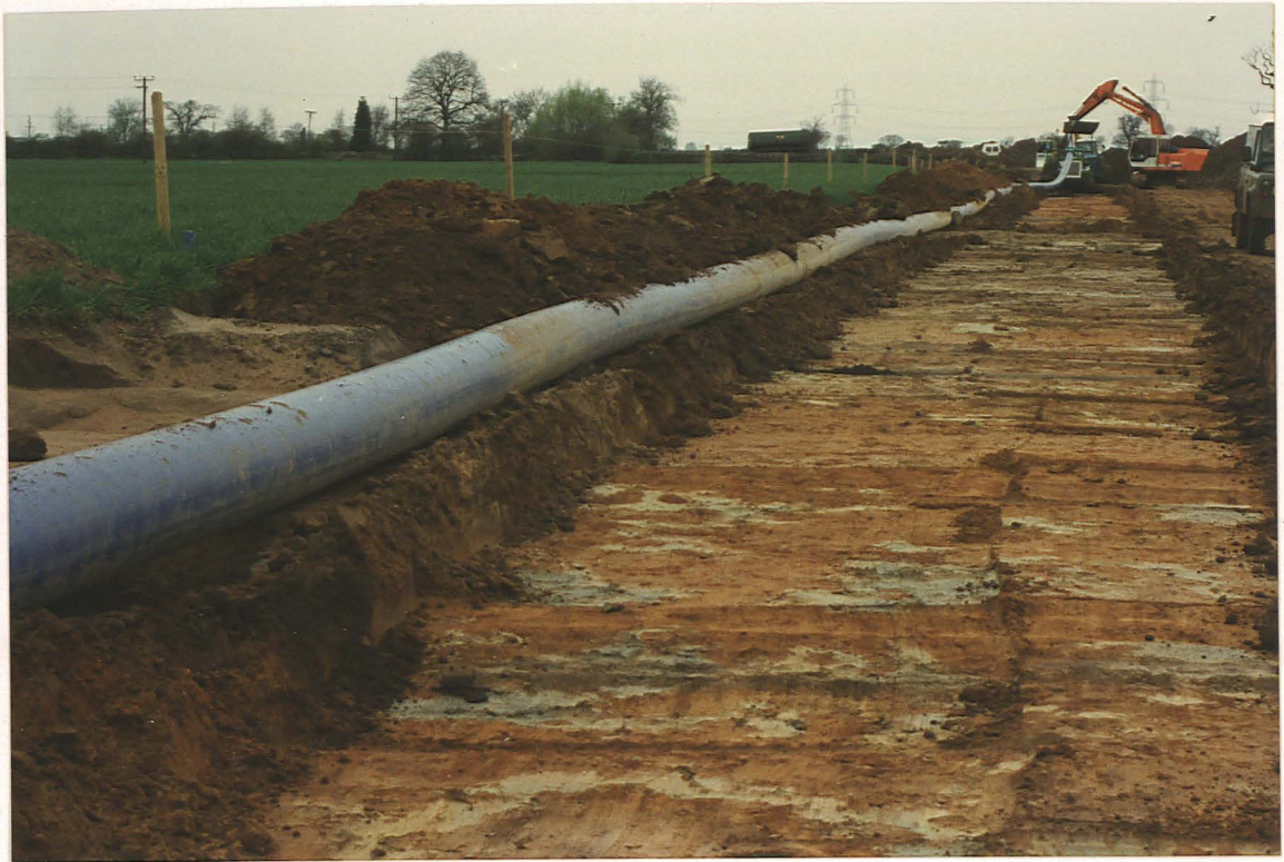
Pl. 41 A ditch crossed the easement in a dip between gully 101 (foreground) and the enclosure entrance (behind trenching machine); the depression is behind the landrover (looking north).
