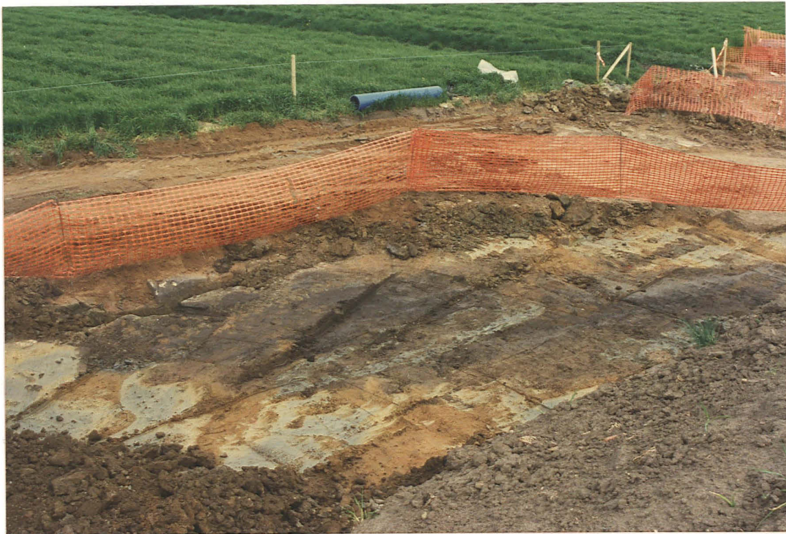
Pl. 27 After diversion of the contractors' access over 308, trample was removed from above ditch 307 by machine. Redeposited grey clay in ruts is still visible (looking NW from spoil heap).
