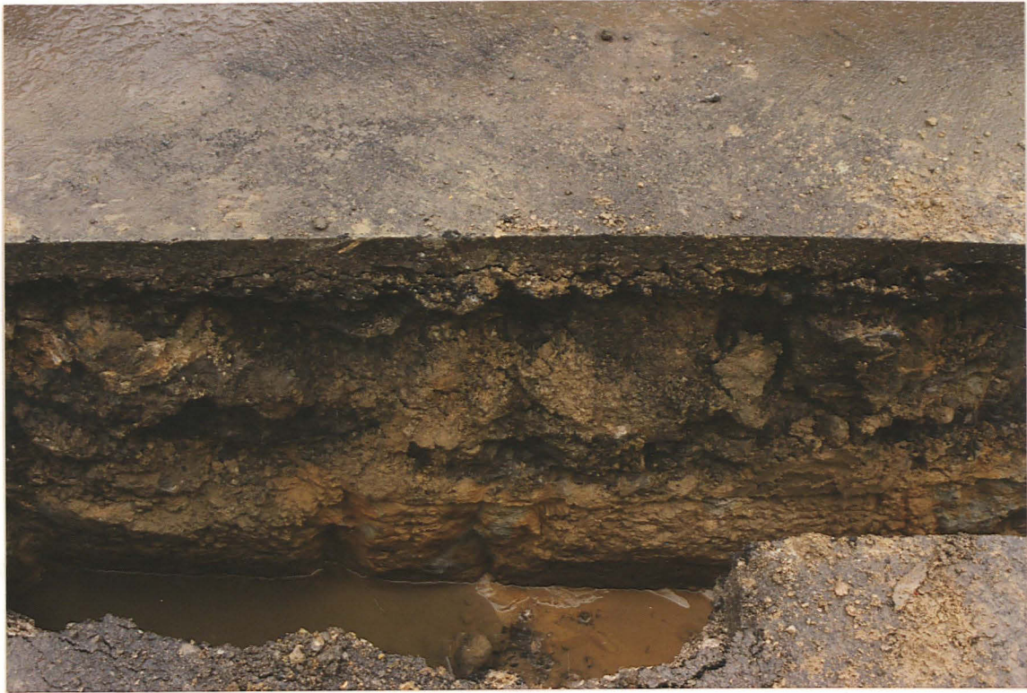
Pl. 3 The trench at 4 revealed thick road foundation material (perhaps in a roadside ditch) overlying black soil. Beneath this were sand flood deposits.
