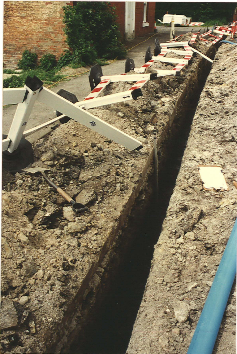
Pl. 10 Location of the peat formation centred between 'Perrin's Cottage' and 'Five Mile House' 13. Looking west past 'Five Mile House'.
