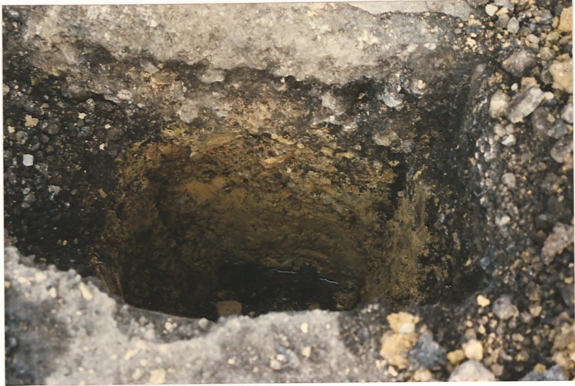
Pl. 17 Small hole excavated for the directionally-drilled pipe at 21, between 'Greengates' and the 'Carpenter's Arms'.
