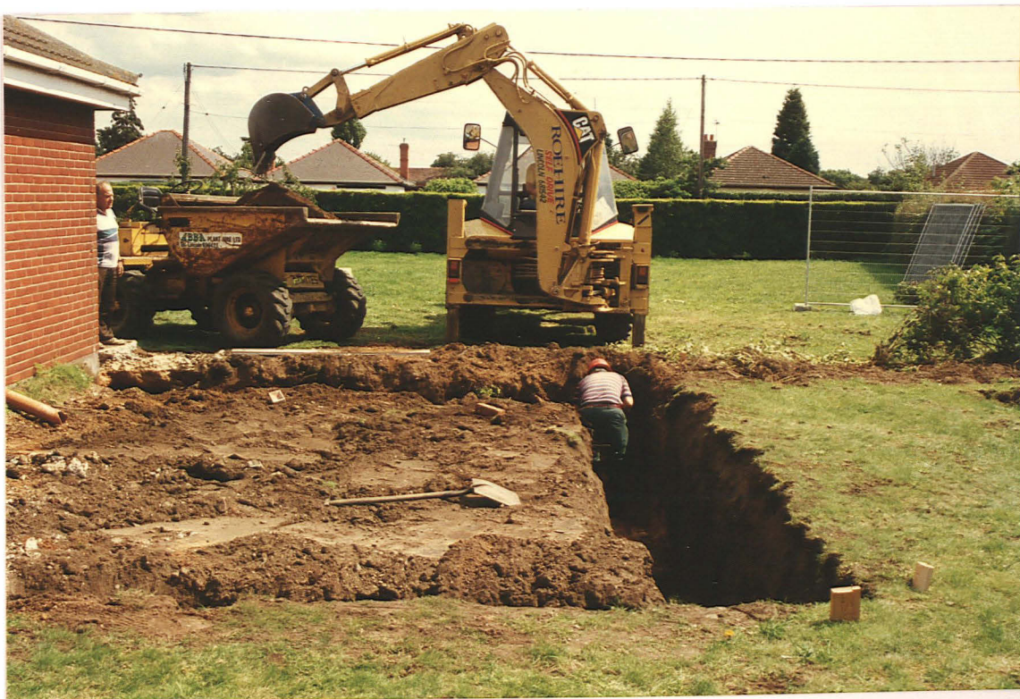
Pl. 2 Excavation of foundations for the extension west of the bungalow (looking south towards Newark Road).
