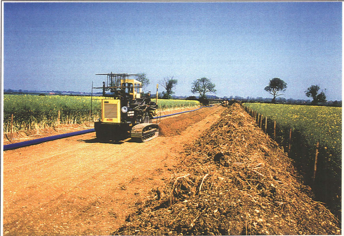
Plate 1: The trenching machine working south along the pipeline easement (Area 3). On a good day this machine could excavate a trench 2m deep, 500mm wide and 1000m in length.
