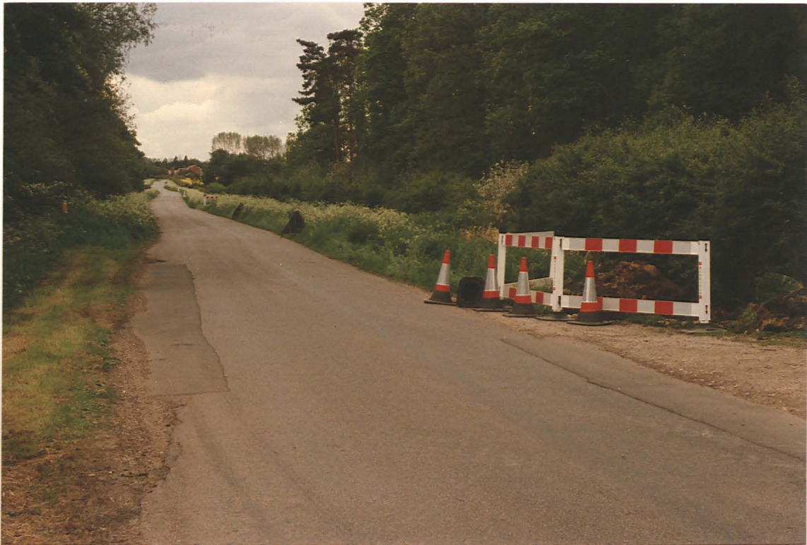
PI. 2 Position of moling access pit 3, beside the entrance to Stixwoud Plantation (looking SW).
