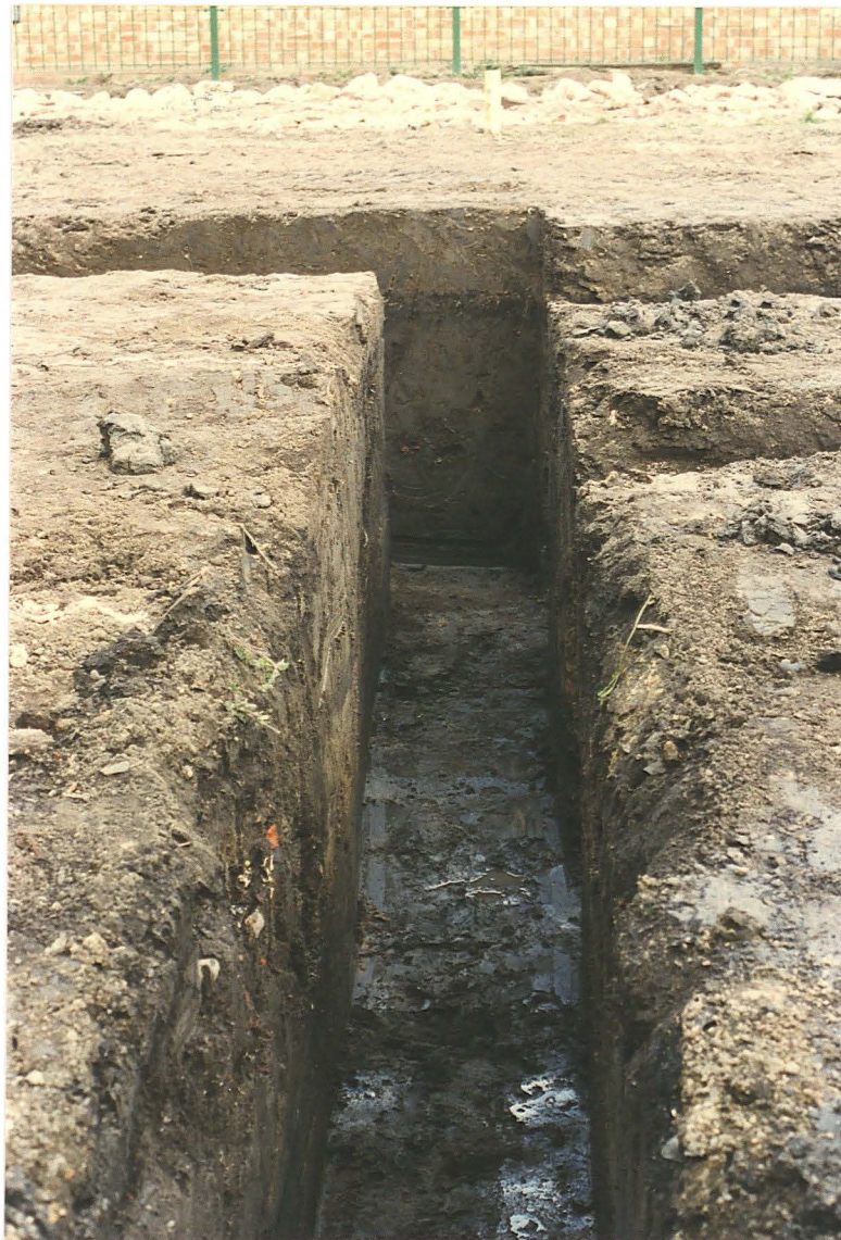
PI 4: The trench for the main back wall of the house, looking north, and showing a typical section through the make-up layers.
