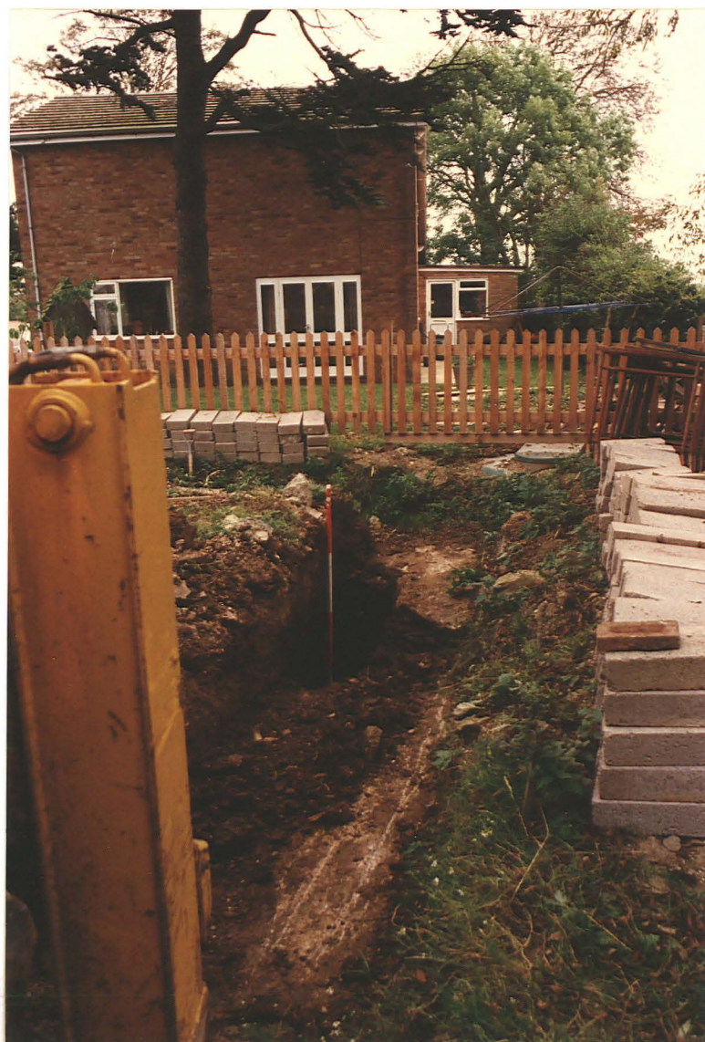
PI. 6 Trench 1, shared septic tank cover below fence. Priory House in background. Tree-lined drainage ditch to right. From west.
