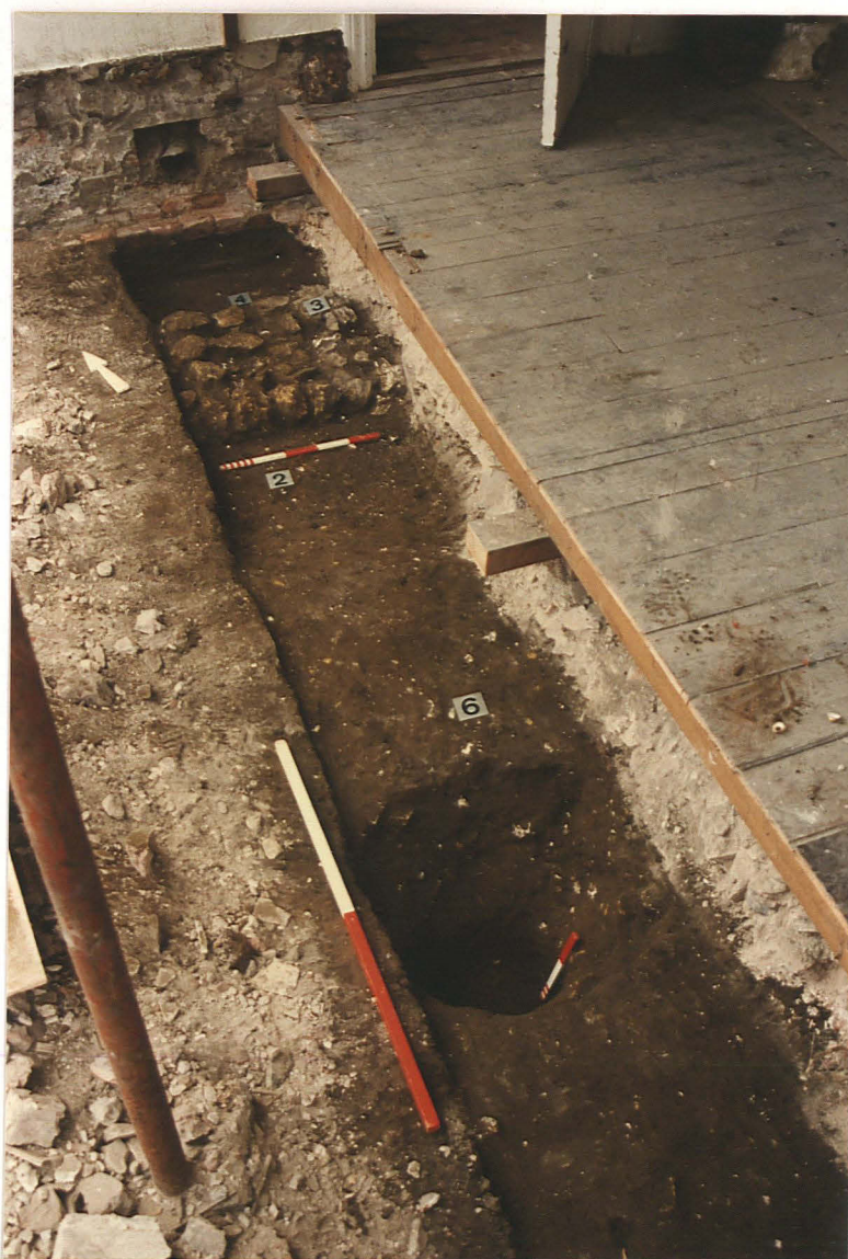
Pl. 4 Foundation trench with scaffolding hole 6 and wall 3. Looking NE. Vertical scale 0.25m, horizontal scales 0.50m and 1m.
