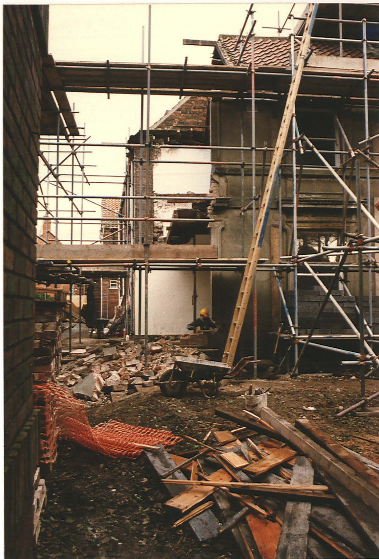
Pl. 1 Casterby. Showing demolished west gable. View NNE.
