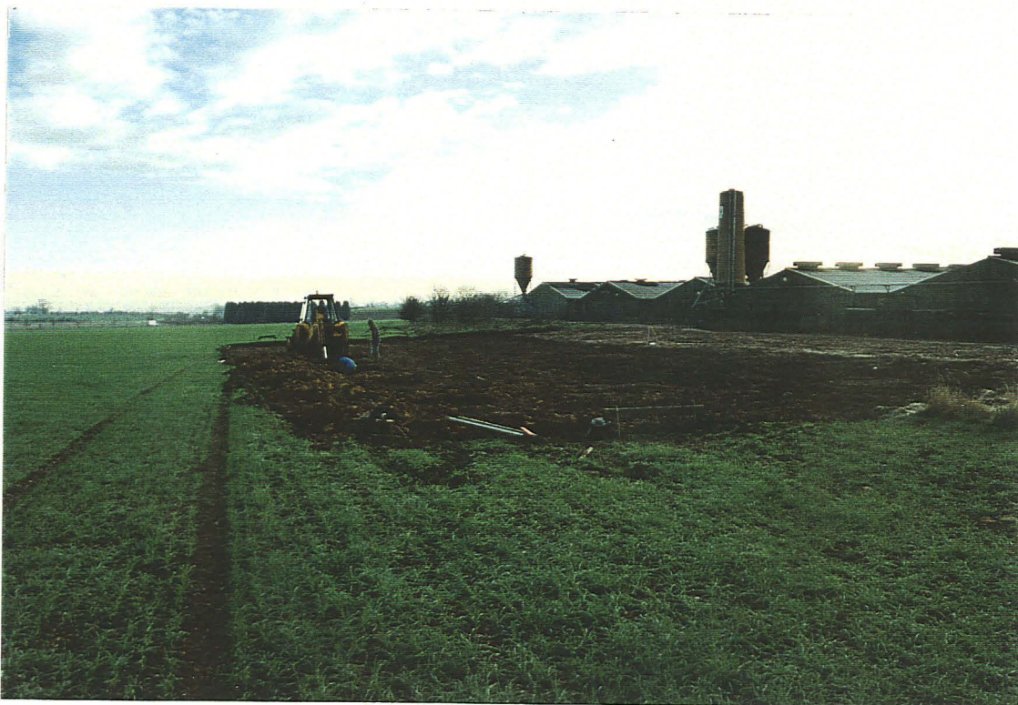
P1 General view of site following soil stripping and during the excavations for north wall of building
