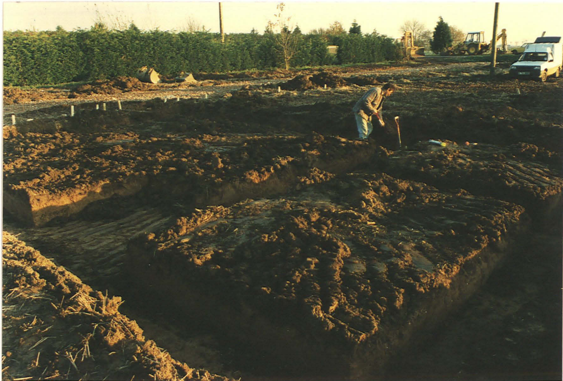
Pl. 2: View of excavated foundation trenches, from centre of back wall, looking south-east.
