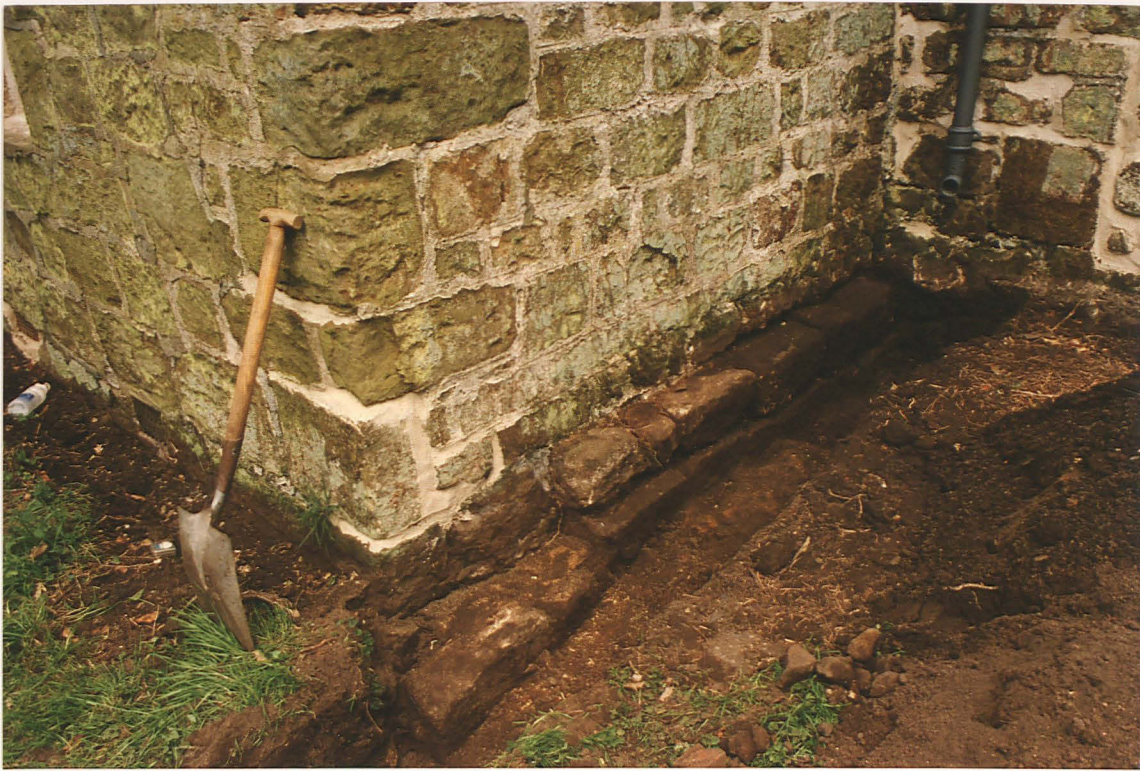
Pl. 11 Trench 5 running along vestry west wall showing two courses of stepped foundations for the vestry overlying foundations of an earlier structure
