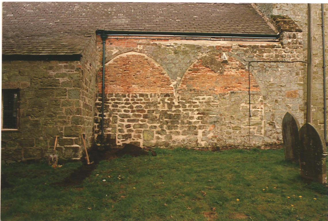
Pl. 10 General view of blocked north aisle arcade with vestry to left, showing Trench 5
