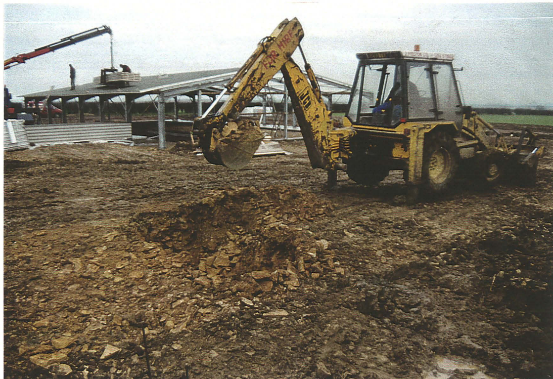
P1 General view of site looking north-east: Shed No. 3 in background, start of waste tank in foreground
