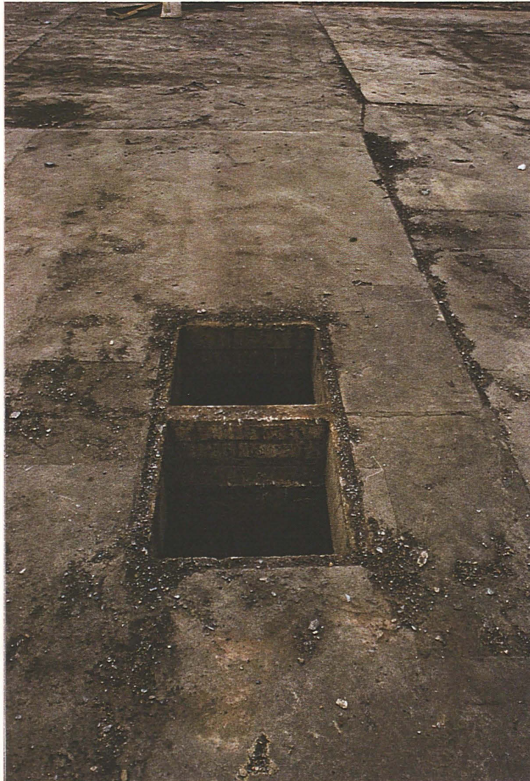
Pl. 4 Inspection hatch over drains of unknown size and extent.
