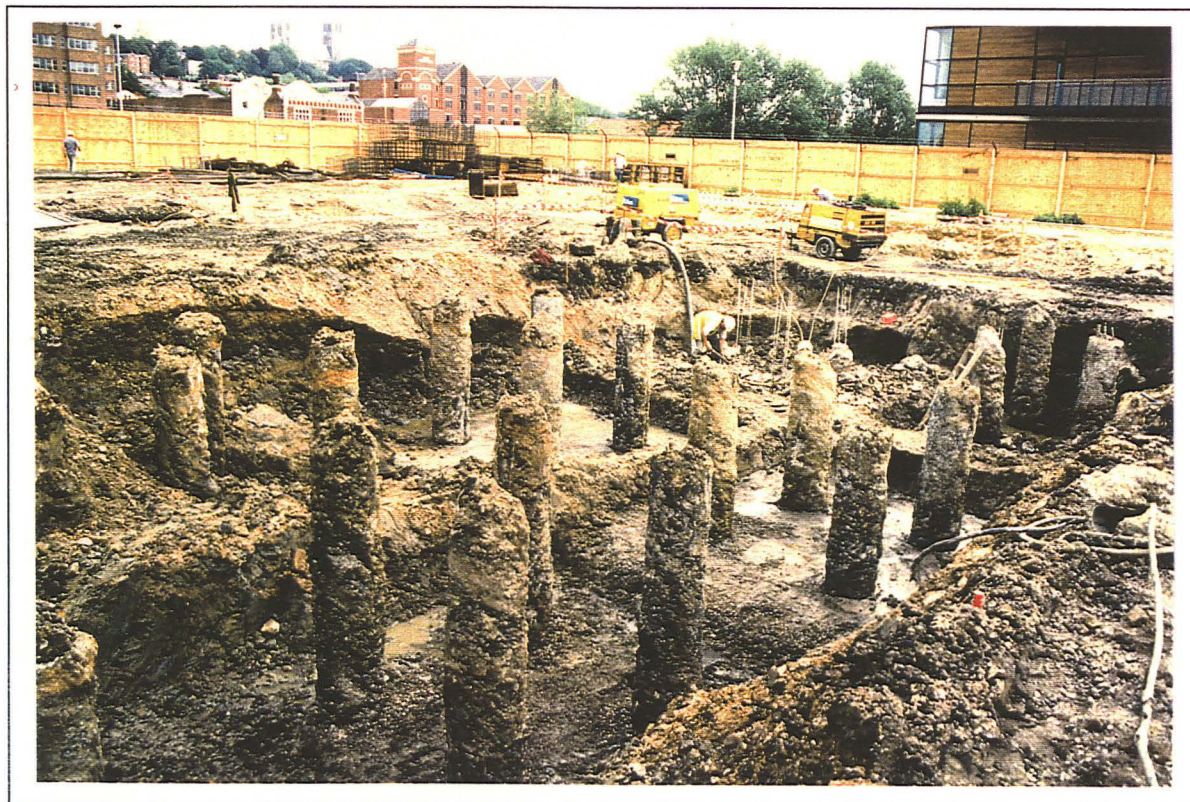
Plate 2: General shot of site conditions during excavation of piles & formation of pile-caps
