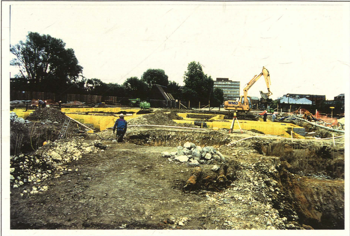
Plate 3: General view of groundworks in progress, during construction of main university building (UCLB95)
