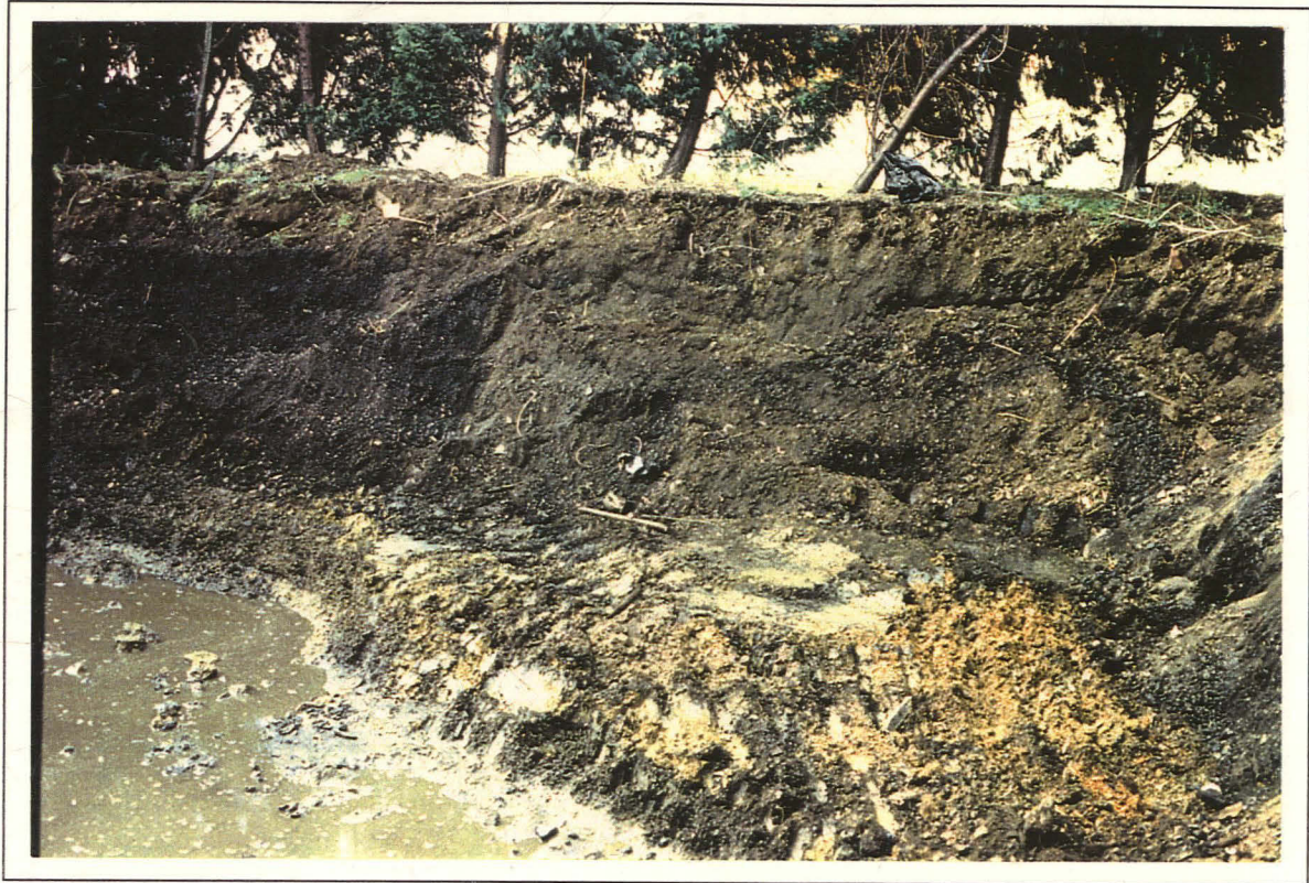
Plate 1: General view of ground conditions, former scrapyard area, Phase I(b) Remediation Works (UCLA95)
