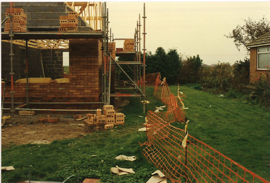
Pl. 2 Northern wall of the bungalow, Plot 10, during construction. The kiln waster material was found in the foundation trench at the NE corner, and Ditch 17 coincided with the northern wall trench. Looking west.
