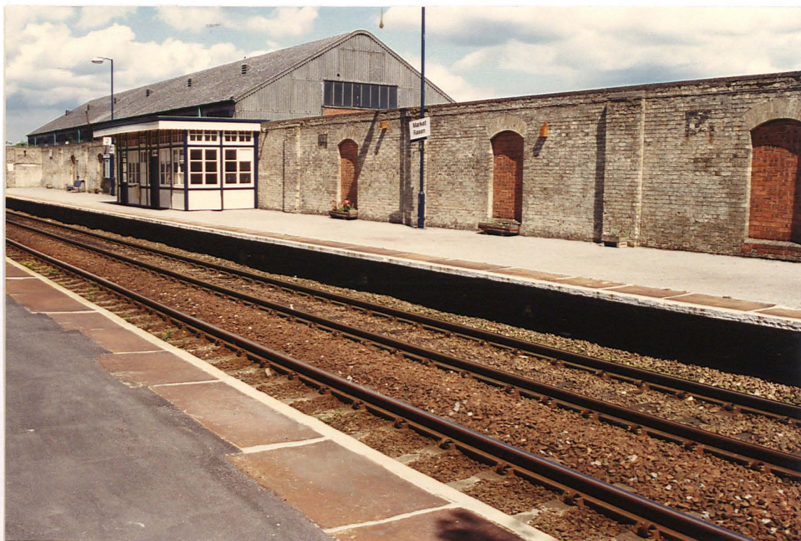
Pl. 2 Wall with brick blockings on eastern station platform (looking NE to the goods shed). The wall supported the train shed roof.
