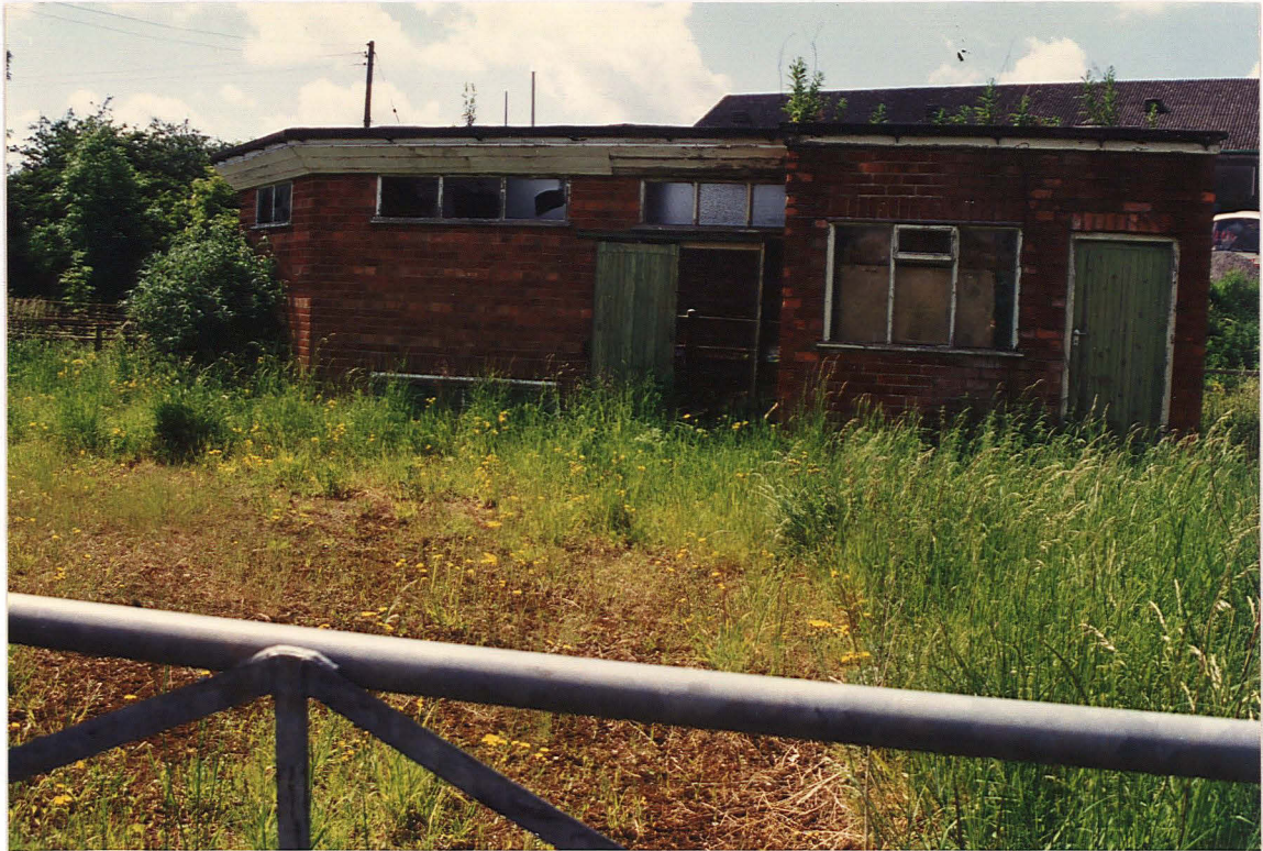
Pl. 6 Derelict cattle market building, with goods shed on higher ground in background. Looking west.
