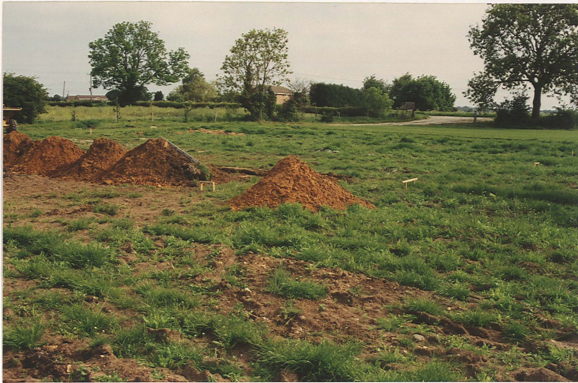
Pl. 1 Location of the monitored groundworks close to the assumed position of the Car Dyke, visible as a depression beside Washingborough Road (looking NE).
