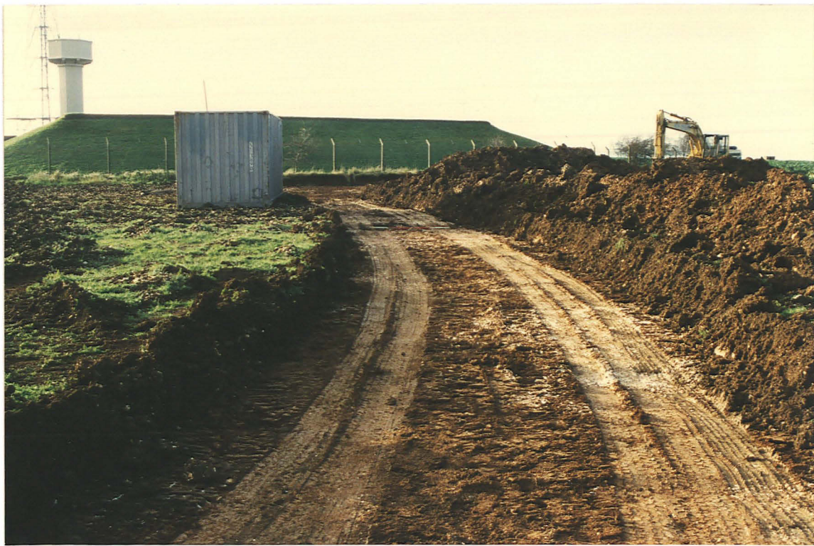
PI. 1 Surface conditions during topsoil stripping for the reservoir extension (looking west to the existing reservoir compound).
