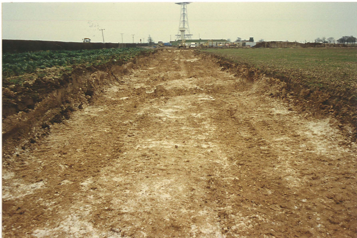
PI. 10 Vehicle ruts in temporary haul road, probably marking positions of archaeological features. Looking SW to new reservoir construction site.
