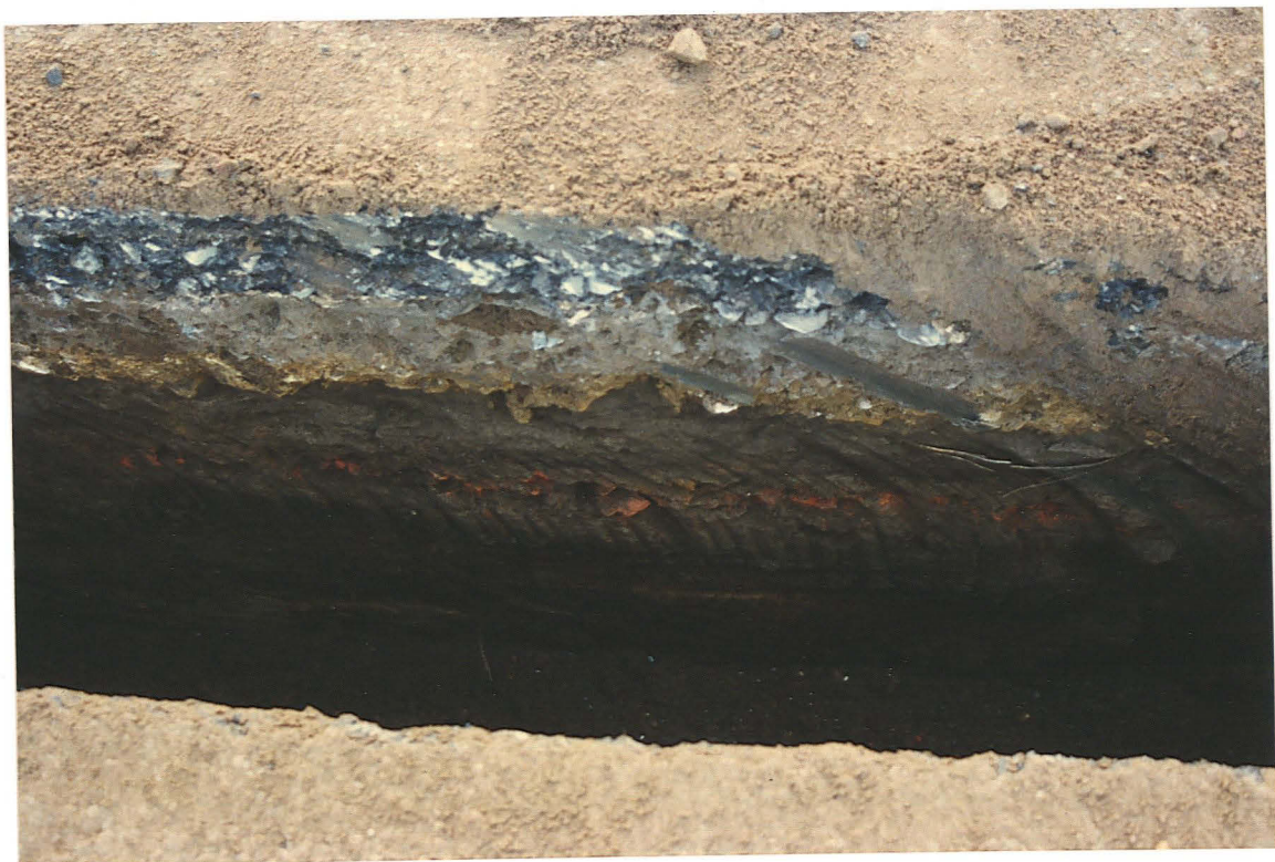
PI. 17 Red clay drain pipe below road, in former roadside ditch, 7H.
