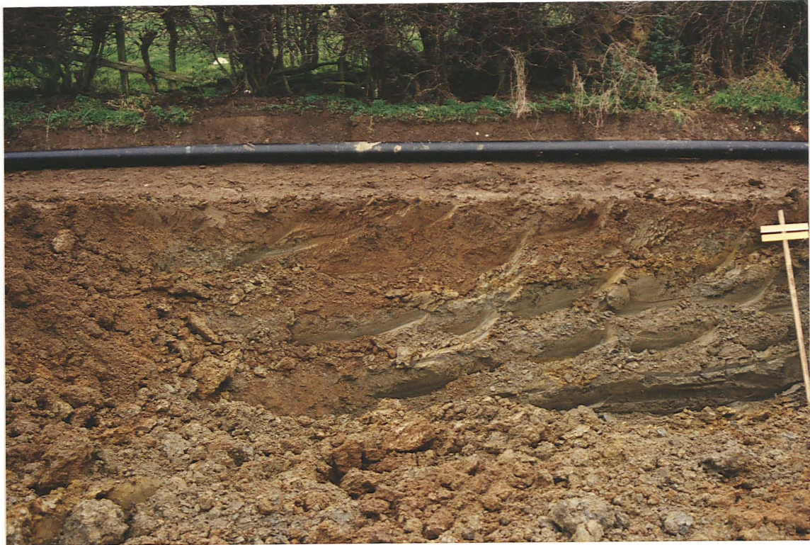
Pl. 5 Brown fill of medieval/post-medieval plough furrow 54 visible in pipe trench face close to field hedge (looking east).
