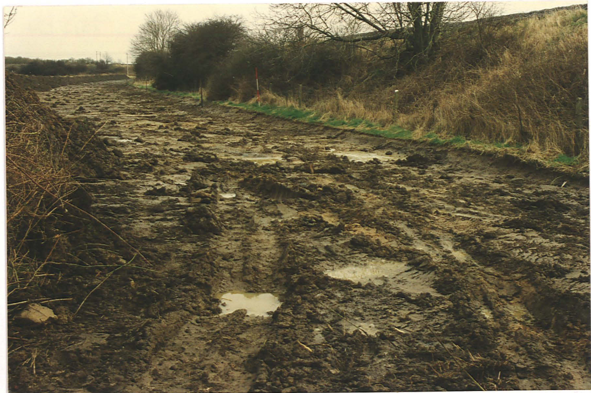
Pl. 19 The pipeline easement north of Sand Lane, with railway to east (looking NE).
