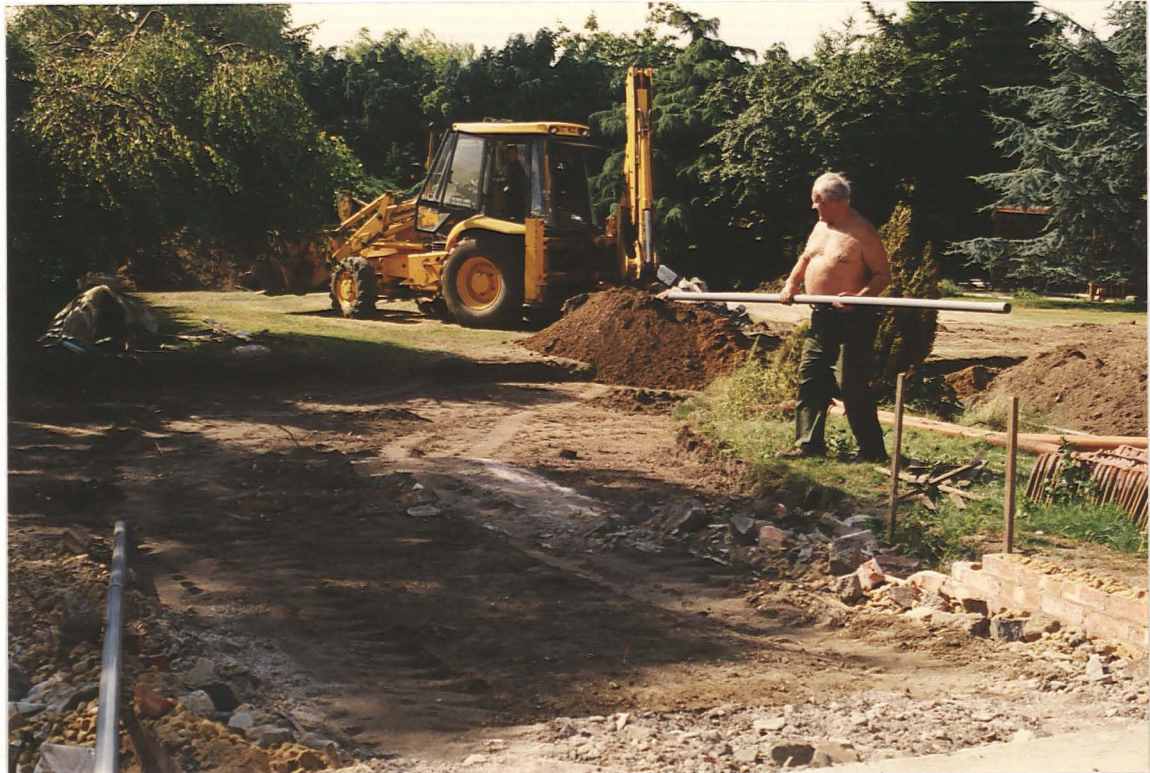
PI. 3 Excavation of the side spur from the service trench (looking west from the demolished garage).
