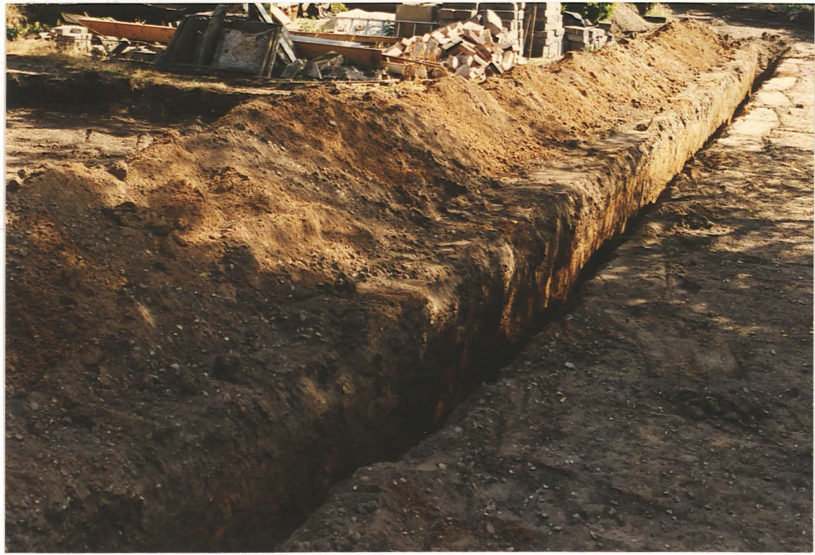
PI. 2 Dark fill of modern disturbance 2 (left foreground) and the new trench for services.
