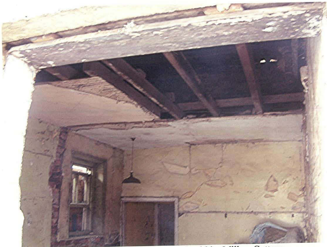
Plate 9. Showing missing floor above Room A within Millers Cottage
