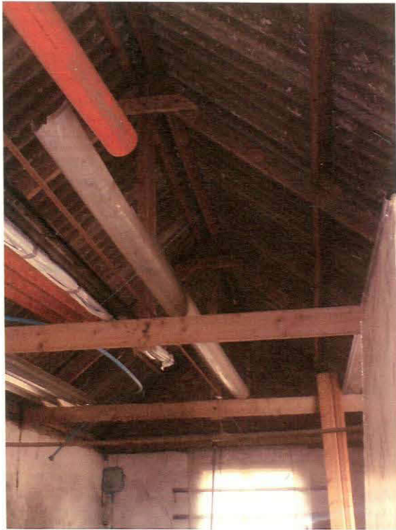
Plate 21. Showing interior of adjoining outbuilding with modern roof timbers and corrugated asbestos sheet roof.
