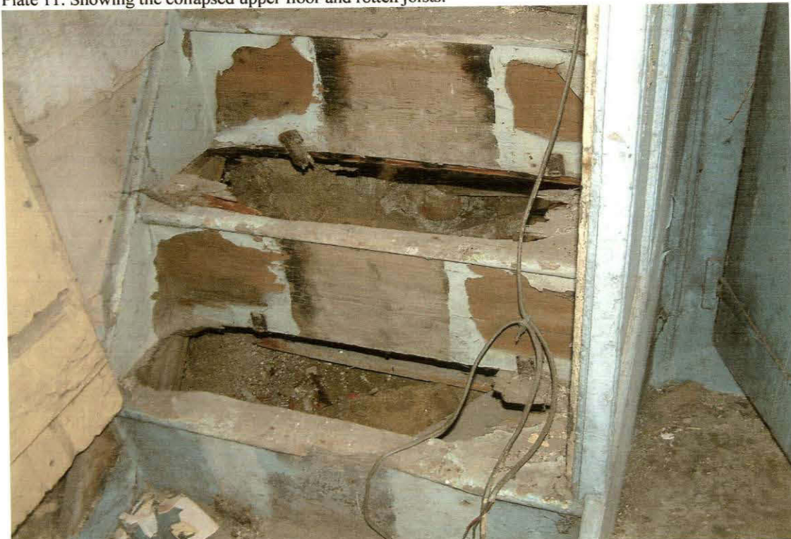
Plate 12. Showing collapsed stair treads apparent all the way to the top of the flight.
