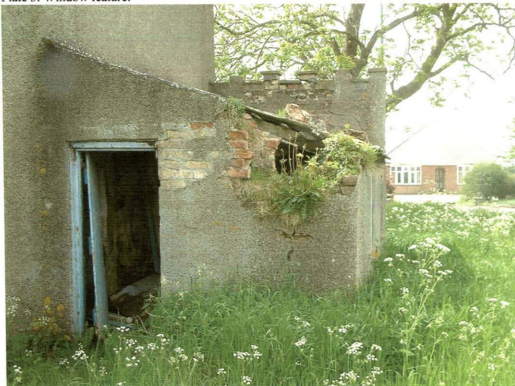
Plate 4. Showing poor condition of roof in extension.
