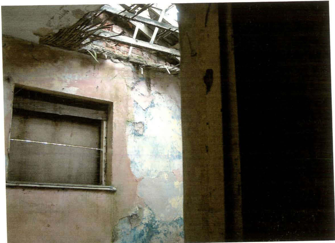
Plate 15. Southern bedroom showing the collapsed in roof and lathe and plaster ceiling
