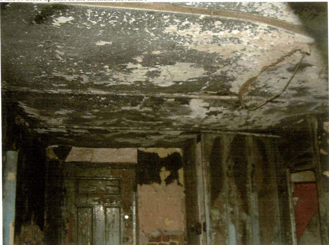
Plate 10. Showing fire damaged ceiling.
