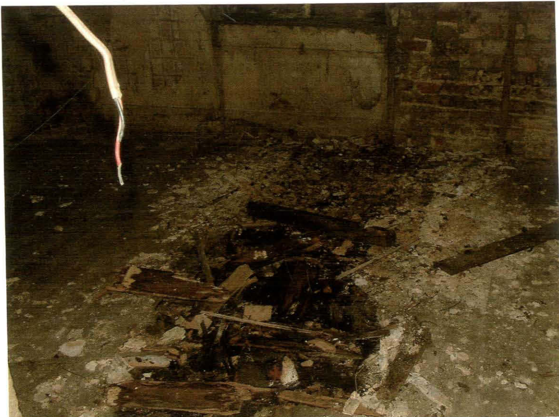
Plate 11. Showing the collapsed upper floor and rotten joists.
