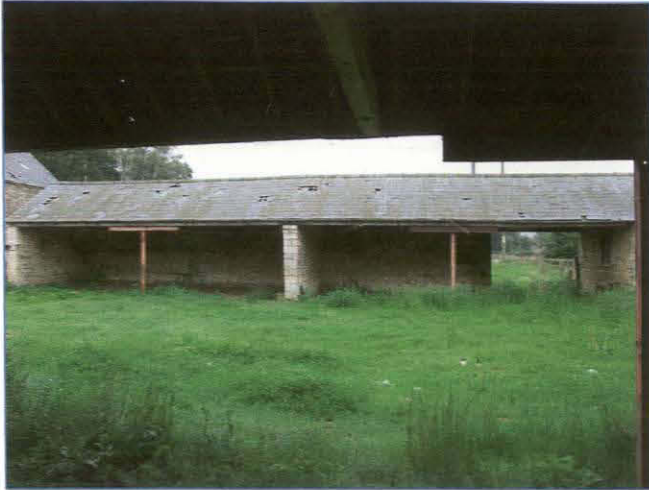
Plate 13: North elevation of cart shed Building D, looking south-south-east. Note the opening at the rear of the building allowing access to the fields beyond.
