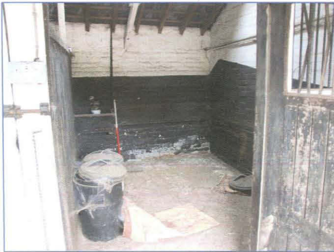
Plate 5: Interior of one of the stable blocks at the north end of Building B. Looking west.
