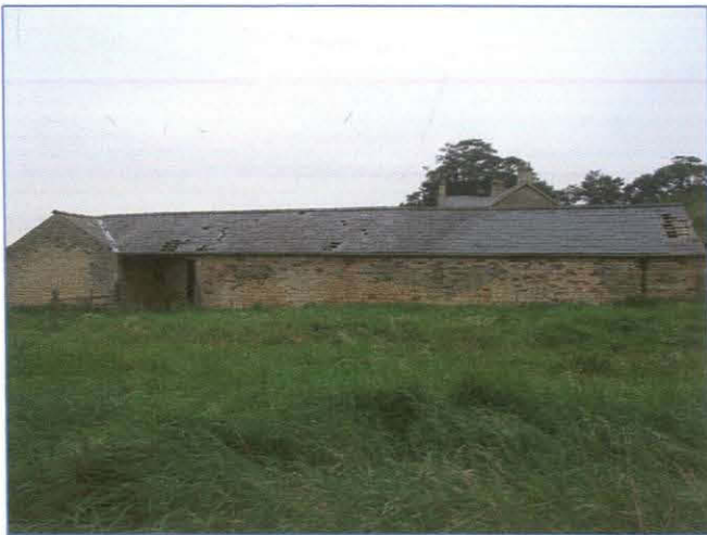
Plate 14: South elevation of cart shed Building D and Building B, looking north-north-west.
