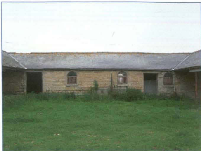
Plate 10: Southern part of the east elevation of Building B, between cart shed Buildings C and D. Looking west-south-west.
