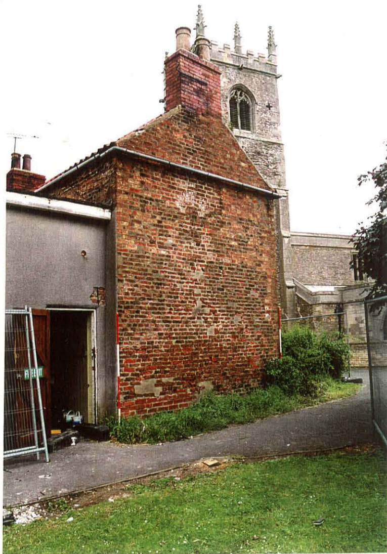
Pl. 3 Gable end of School House, prior to demolition of reading room. Looking N.
