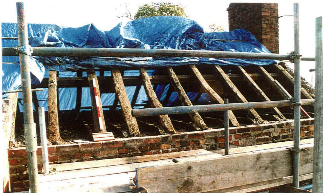
Pl. 10 Roof timbers exposed after removal of the School House roof tiles, looking E.
