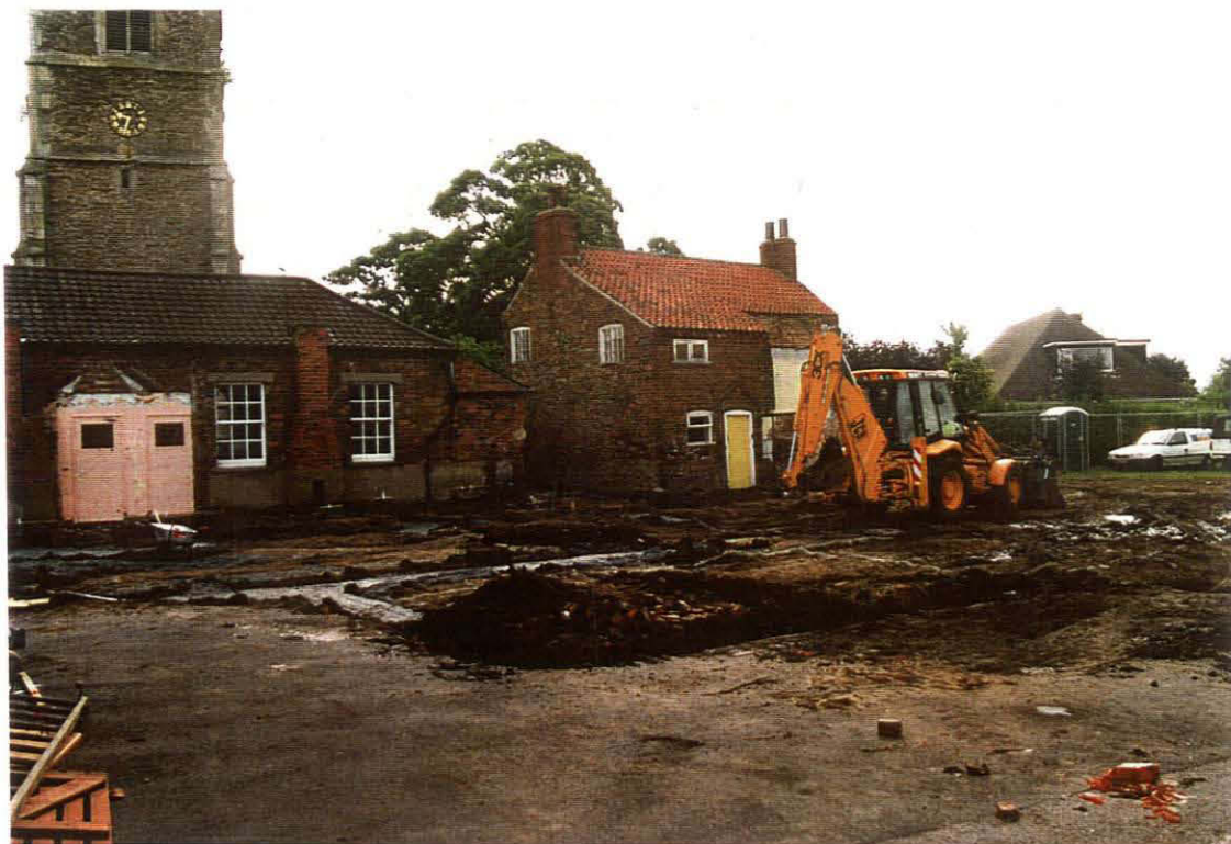
Pl. 12 View of groundworks in playground, looking E. School House (right), Victorian classroom (left), and church tower (background) are visible.
