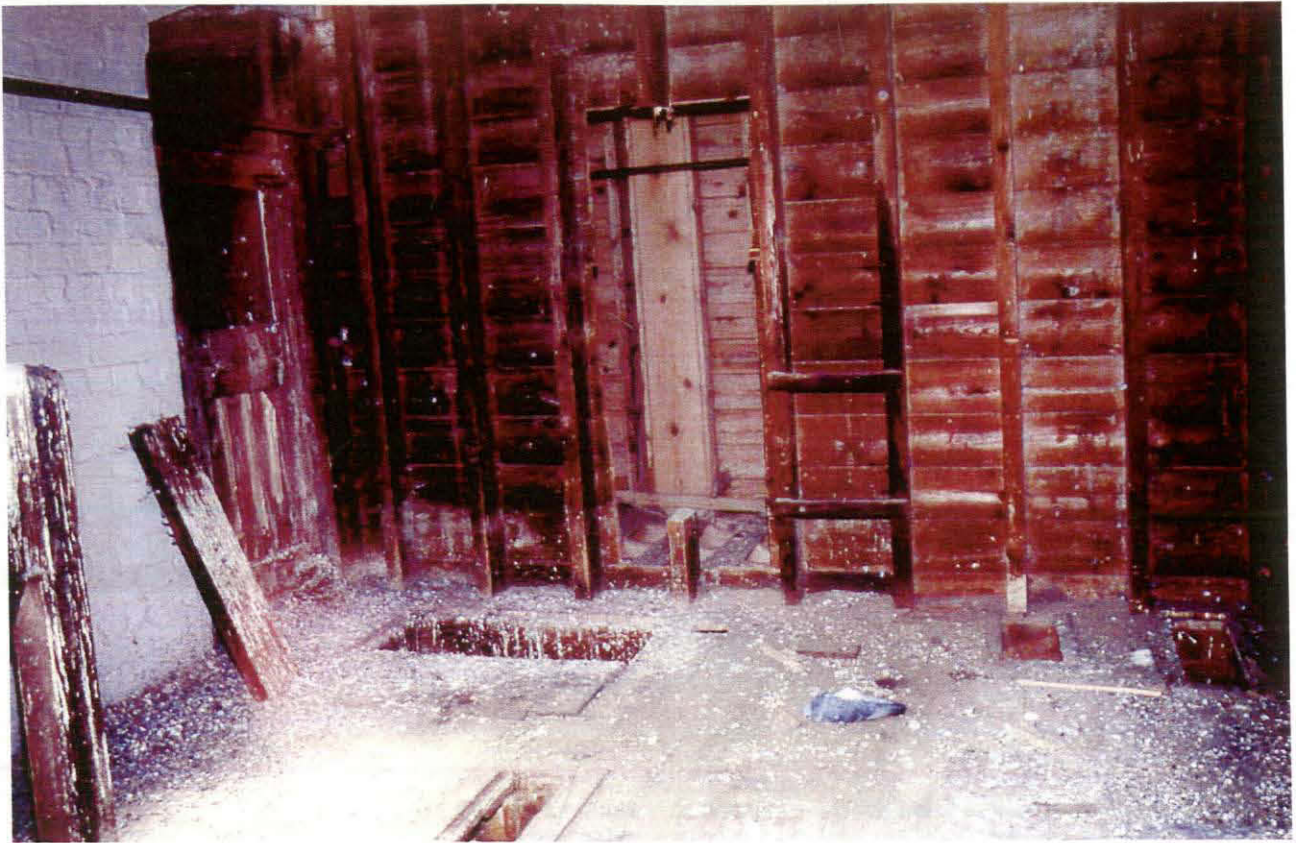
Plate 21 Mill southern part, 4 th storey, showing trap door for sack hoist and elevator ducts
