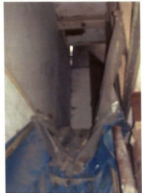
Plate 15 Assessed Building, stairwell up from ground floor, showing separating walls, looking west
