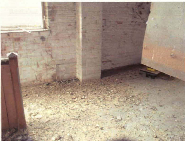
Plate 14 Assessed Building, 2 nd floor, west side, showing blocked window crossed by floor and plinth, looking west
