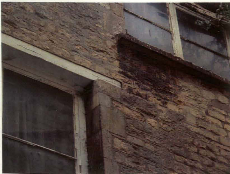
Plate 4 Assessed Building, eastern elevation showing straight join and offset of wall, looking northwest
