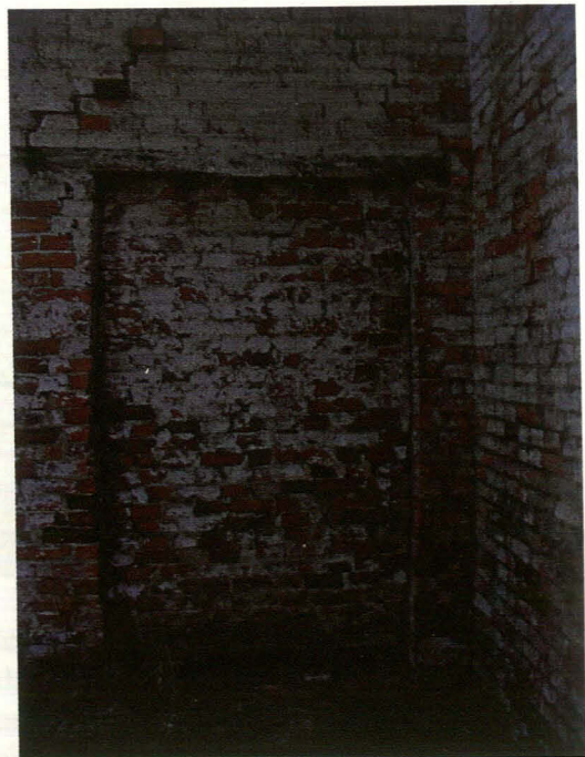
Plate 15 Interior of main barn, detail of east facing elevation, west wall, showing blocked doorway, looking west
