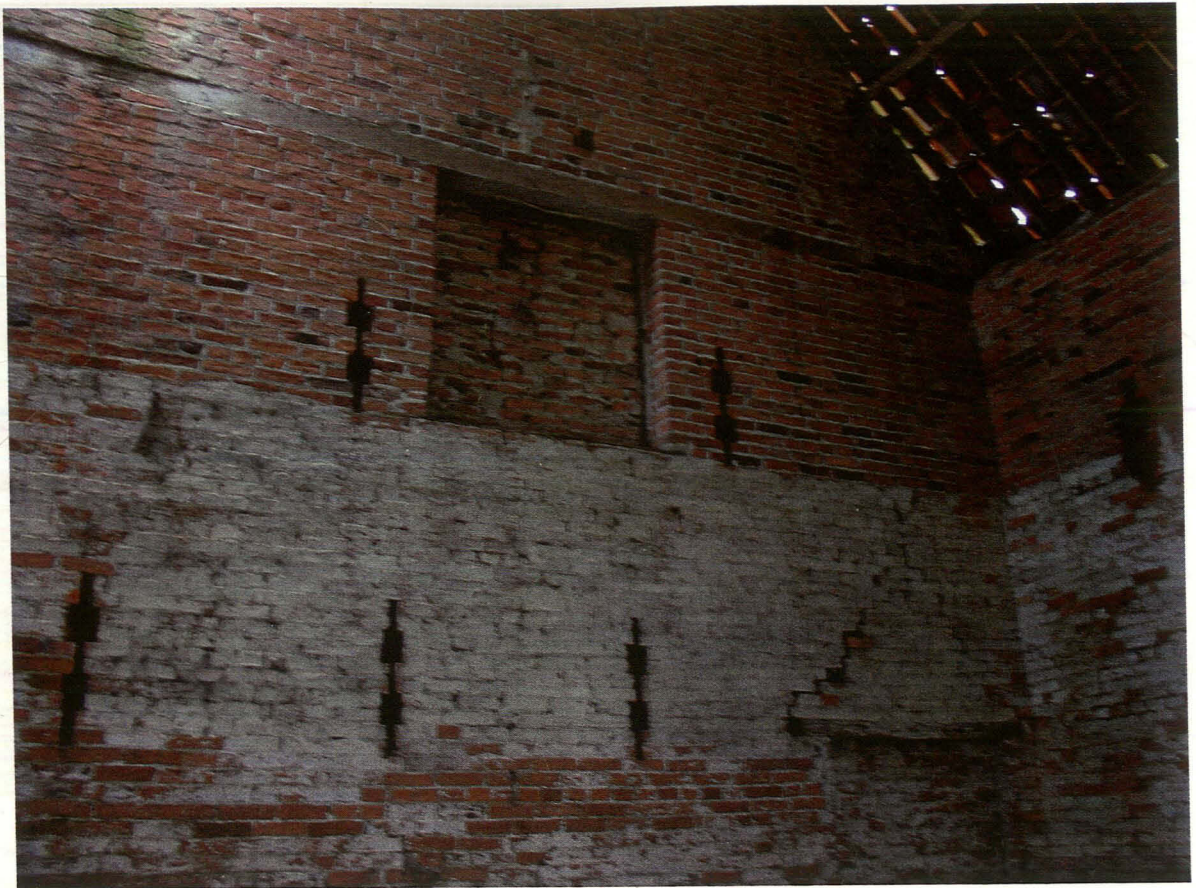
Plate 14 Interior of main barn, east facing elevation, west wall, showing breather slits, blocked window or pitching hole and blocked doorway, looking northwest
