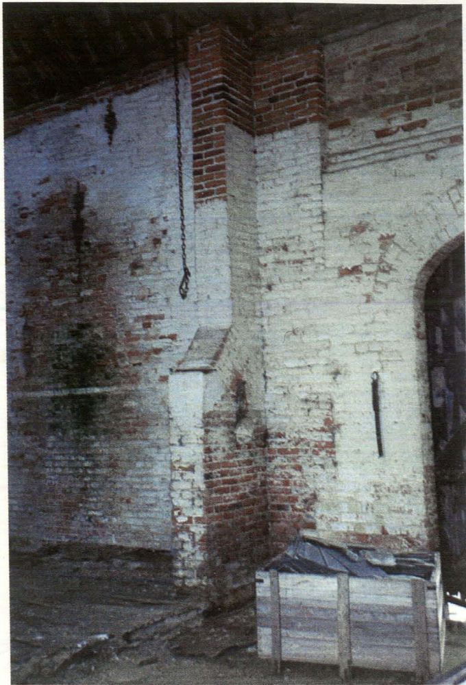
Plate 20 Interior of main barn detail showing infill around east side of southern doorway and plinth construction of barn, looking southeast
