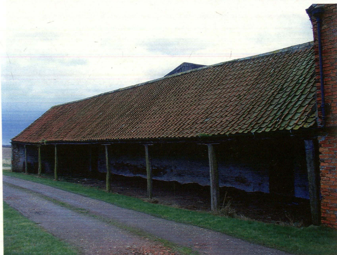
Plate 30 North elevation of shelter/cart shed at northeast corner of range, looking southeast
