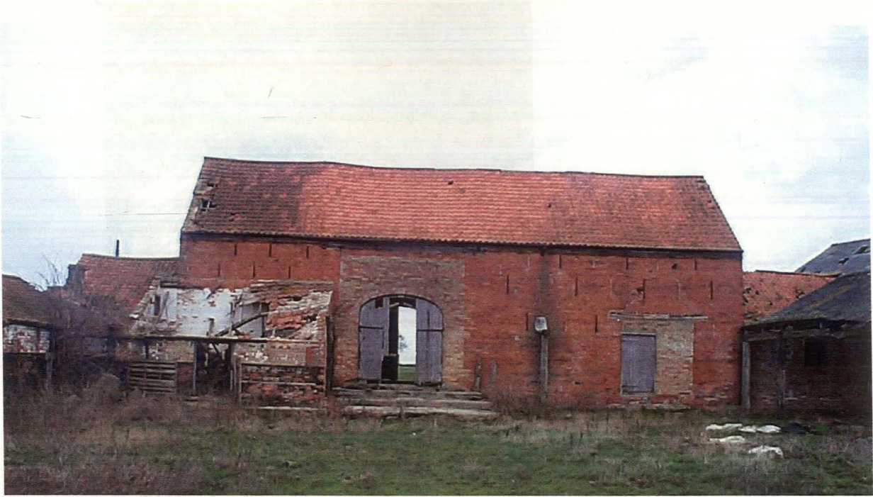
Plate 9 South elevation of main barn including lean-to stable with collapsed roof at left, looking north
