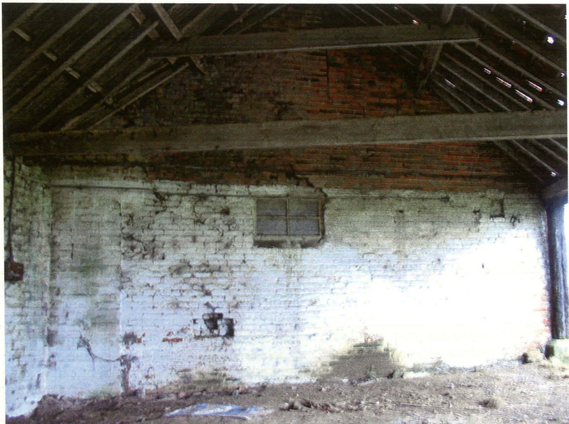
Plate 32 Shelter/cart shed at northeast corner of range, east facing internal elevation (and external elevation of northwest-southeast range), showing blocked window at top, window, blocked niche at right and rebuilt section of wall at left, looking west
