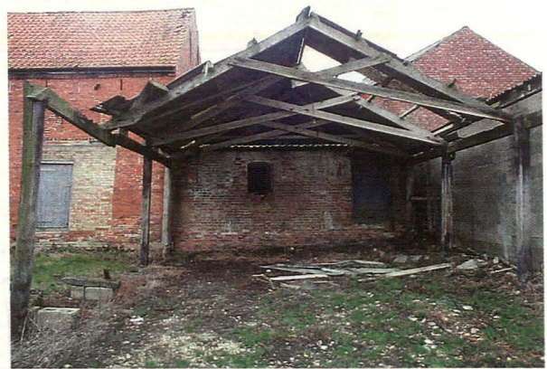
Plate 11 Open-sided shelter forming part of yard covering, blocked doorway in south elevation of main barn at left, window to garage at the centre and door of single storey roofed passageway at right, looking north
