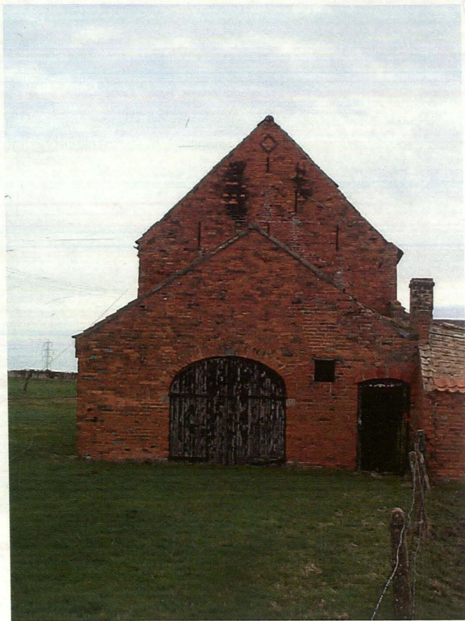
Plate 27 West elevation of main barn and western addition to main barn, comprising possible shed and loose box, looking east
