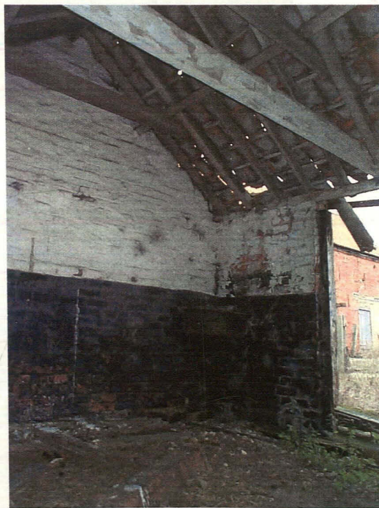
Plate 23 Interior of loose box at centre of western north-south range, showing roof construction, with feed trough just visible in corner of room, looking northeast
