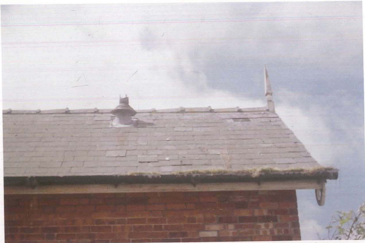
Pl. 14 The roof, finial, guttering and chimney flue on the eastern side of the signal box
