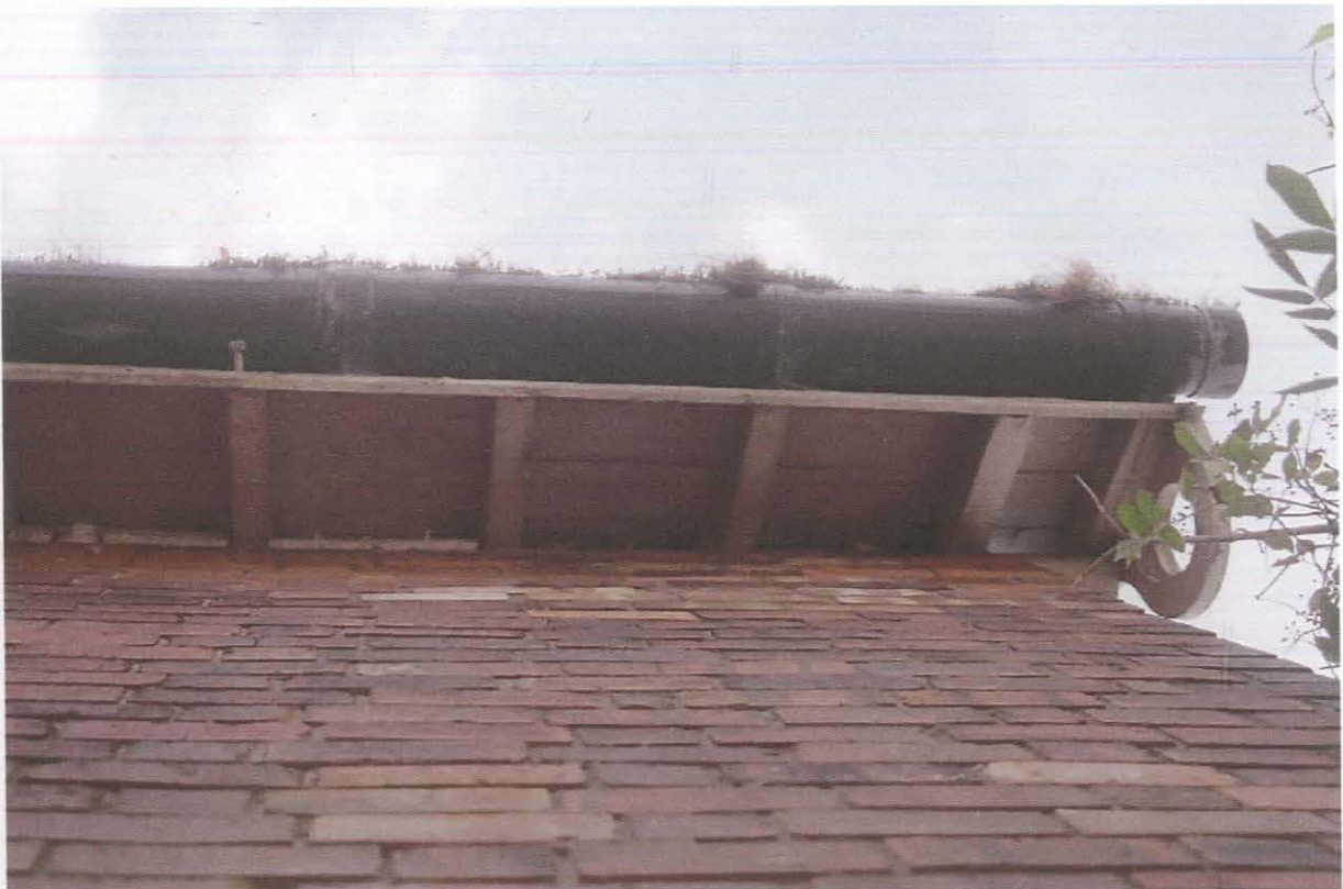
Pl. 12 A detailed view of the underside of the eaves on the north-eastern corner of the building
