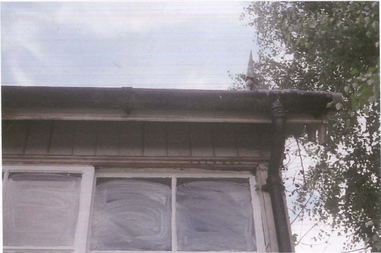
Pl. 11 A detail view of the south western corner of the signal box showing the cast iron guttering and the eaves of the roof
