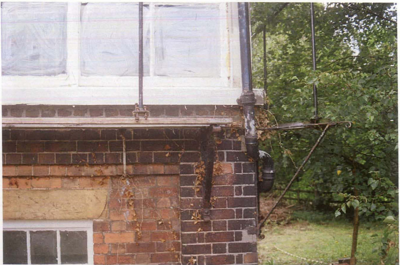
Pl. 4 The west elevation detail showing the cast iron down pipes, recessed window, glazing and balcony on the south-western corner of the building.
