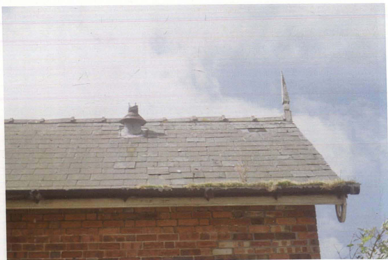
Pl. 2 The roof, finial, guttering and chimney flue on the eastern side of the signal box
