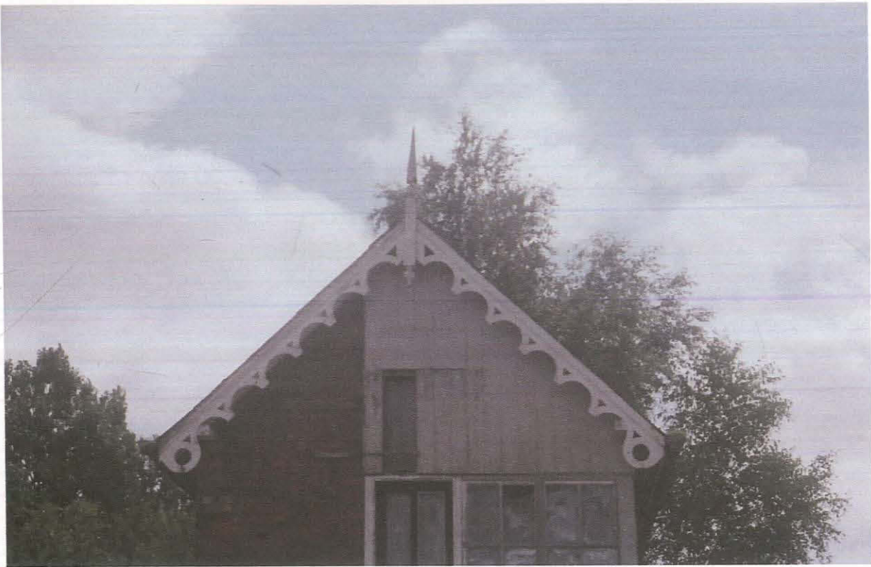
Pl. 15 Detail of the ornate gable end and tongue and grove planking on the northern face of the building
