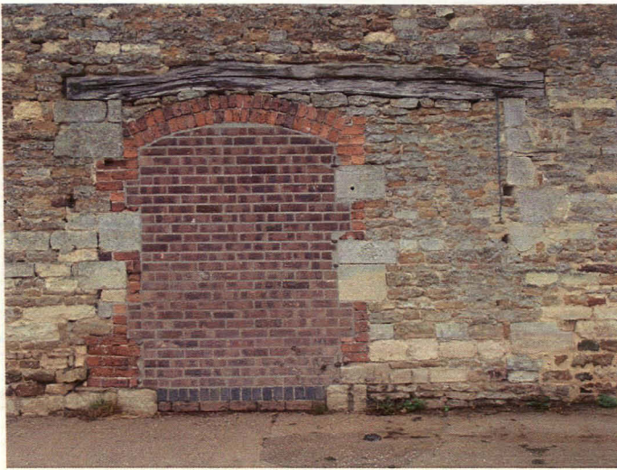
Plate 20 Blocked access in southwestern elevation of southern central barn, looking northeast
