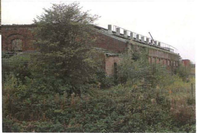
Pl. 4 General view of the engine shed N and E elevations (looking SE)
