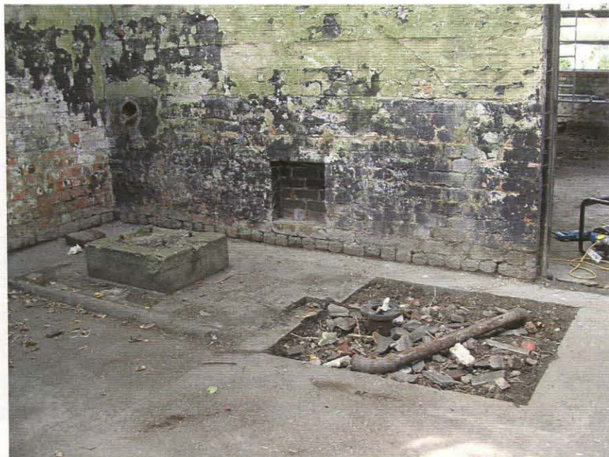
Pl. 32 Water tower interior, oil room, tank base at S end of room
