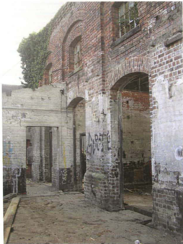
Pl. 25 East extension interior looking S with water tower east wall openings to the right
