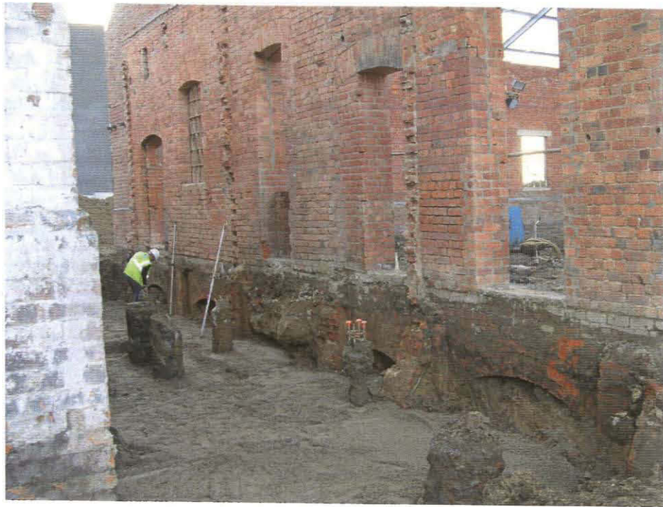
Pl. 37 Groundworks west of the water tower (on site of the west extension, showing the brick relieving arches at ground level (looking north)
