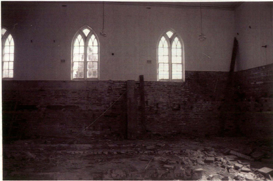
Plate 10 Church interior, east side, showing scars of removed panelling and pews, looking east
