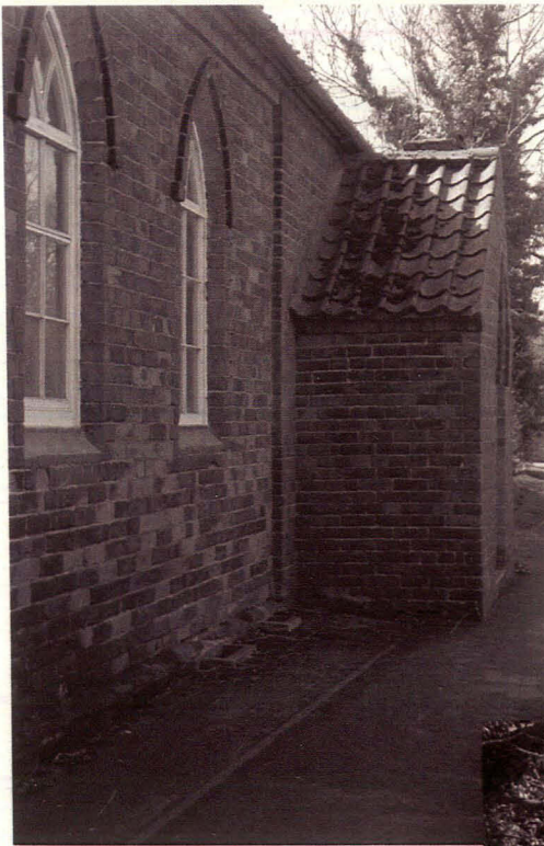
Plate 17 School north side, showing straight join between chapel and school, looking west
