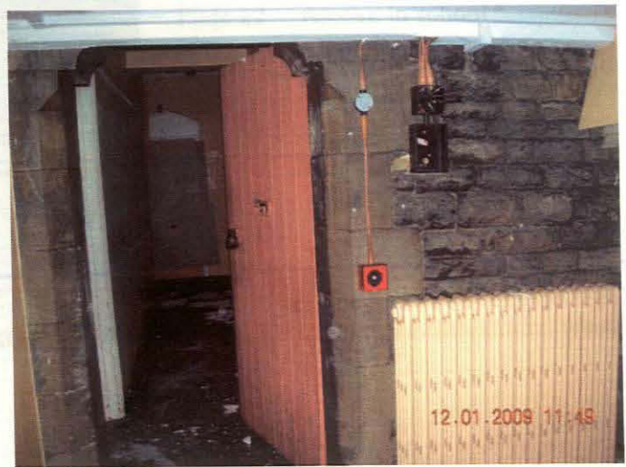
Plate 19 Original external door - door to corridor and view down corridor, looking west
