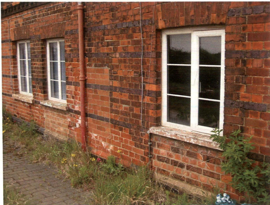
Plate 9 Blocks 3 (left) and 4 (right), southern elevation, showing windows inserted into blocked doorways, and infilled niche, looking northwest
