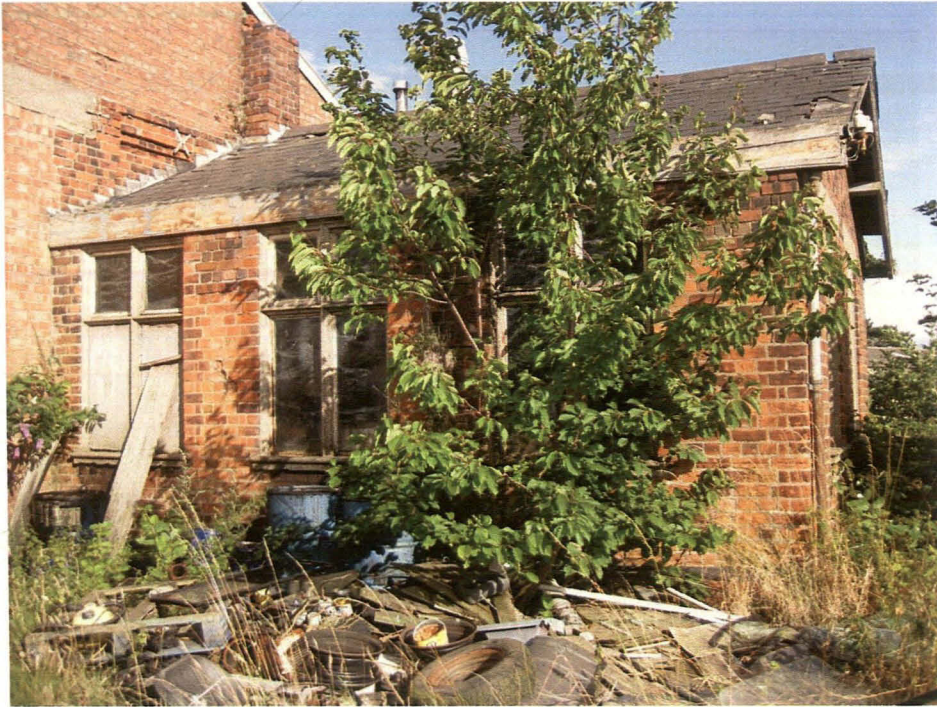
Plate 30 Northern elevation of Block 2. Note recessed panel in wall of Block 1 (on left) crossed by roof line, looking southeast
