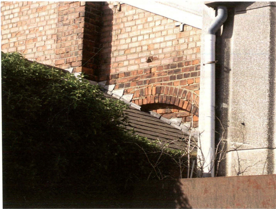
Plate 28 Southwestern elevation of goods shed, showing arched recess crossed by roof of adjacent Block 2, looking northeast
