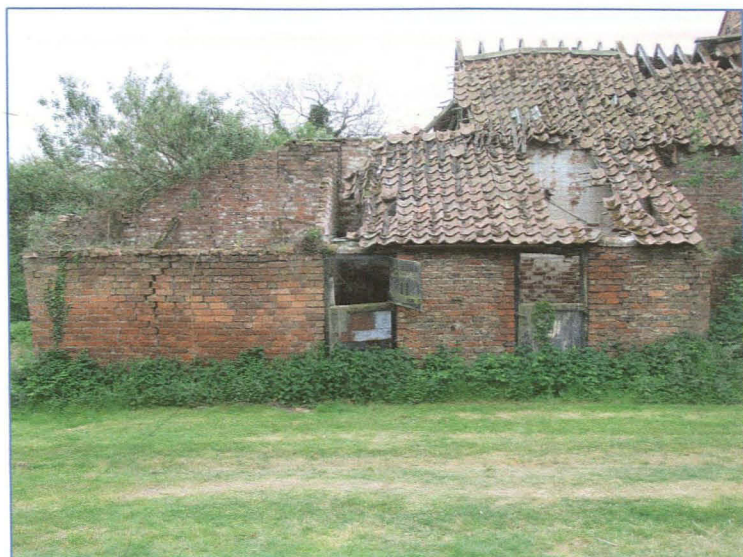
Plate 4: Stable block and cartshed at the east end of the north elevation of the north range. Looking south-south-east.
