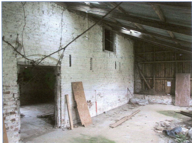
Plate 10: Interior of lean-to on north elevation of north range, showing the door and pitching hole in the north elevation of the barn.
