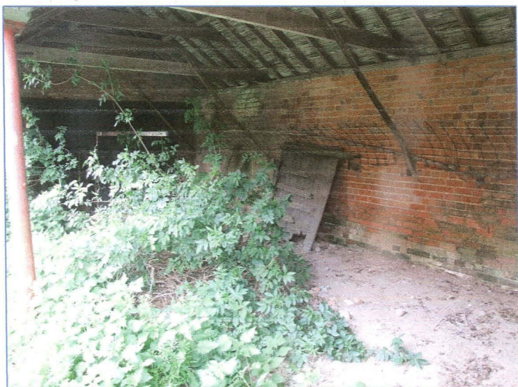
Plate 23: Interior of the eastern bay in the south range, with the feeding rack along the south wall. Looking east
