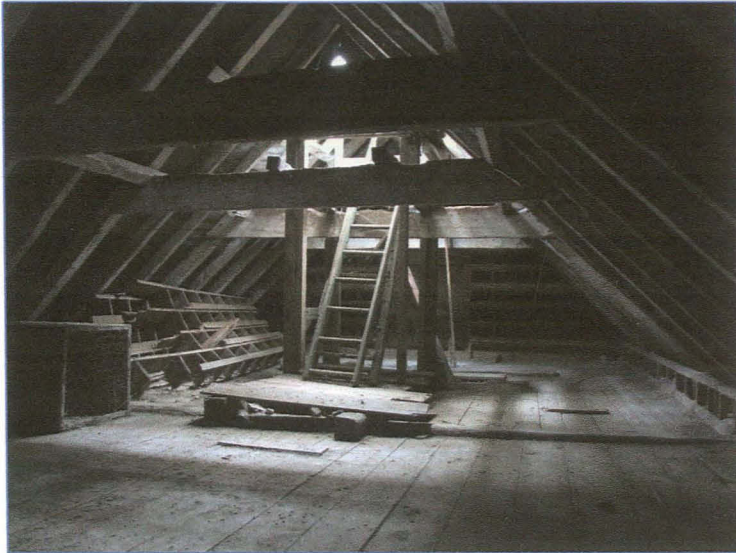
Plate 13: Pigeon cote in the second storey of the threshing barn. Note the pigeon holes at the far end of the room and along the right hand side of the shot, and the ladder allowing access to the cupola above. Looking west.
