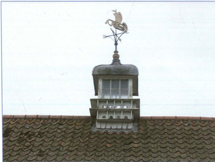
Plate 14: The glazed cupola on the roof of the three storey barn, with the wind vane and flight holes for pigeons. Looking south-south-east.
