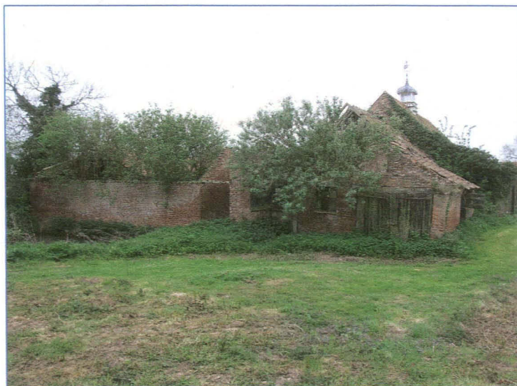
Plate 3: East elevation of the north range, showing the derelict stable and cartshed with the double wooden doors. Looking south-west.
