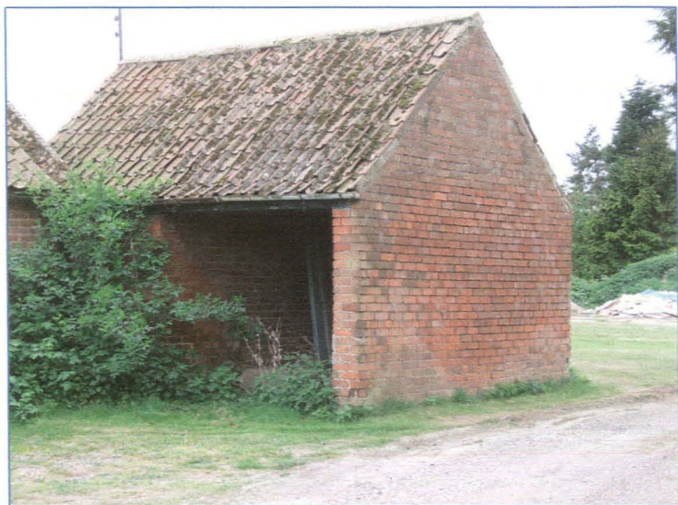
Plate 18: Outbuilding at the east end of the north range, showing the compartment probably used as a cartshed. Looking south-west.
