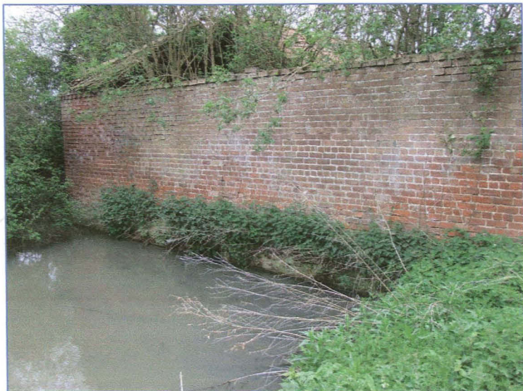
Plate 19: East elevation of the derelict barn at the east end of the south elevation. Looking south.
