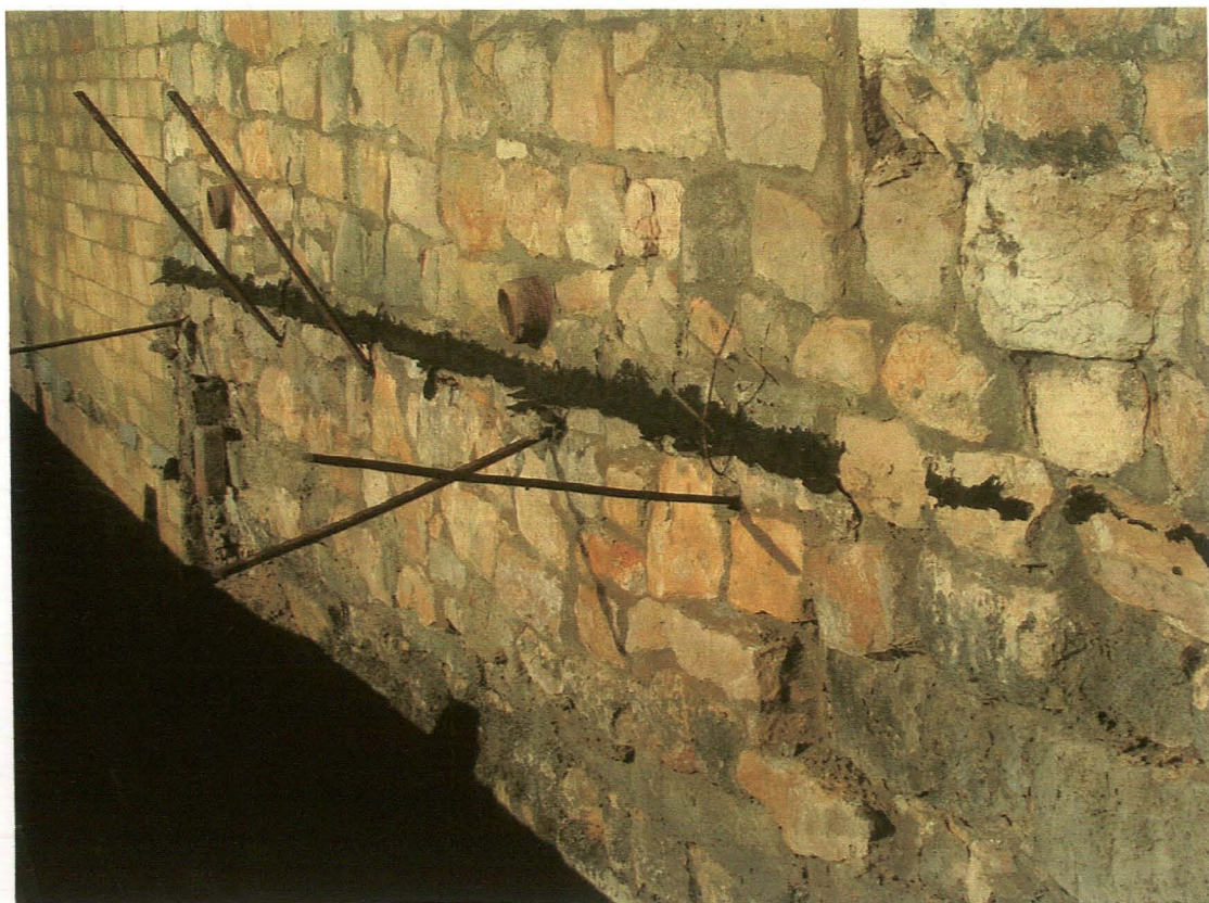
Pl. 6. Bitumen sealant, 100, adhered to Close Wall
