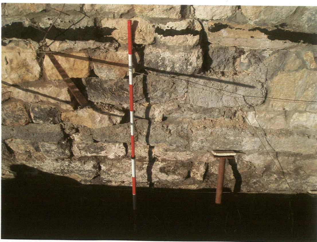
Pl. 8. Detail of medieval fabric of lower Close Wall 103. Looking north. 2m scale
