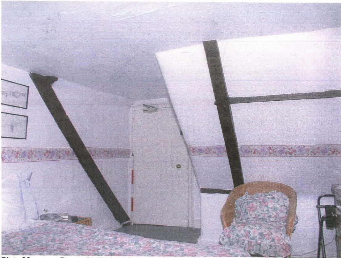
Plate 29 Room 64 (Unit 1) showing cut through purlins to allow entry, taken from the south-west (172)
