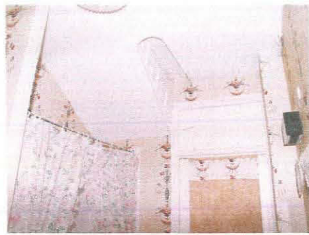
16. Stair line visible in the ceiling of Room 5 (Unit 1), showing the west wall inserted, taken from the east
