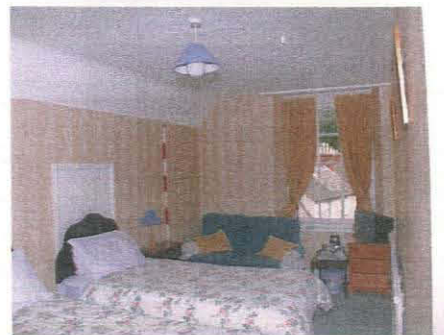
170. Room 65 (Unit 1) showing small sealed doorway leading to the roof space, taken from the south-west
