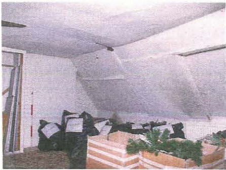
145. Room 68 (Unit 4) showing joggled purlins, butt-jointed to the rafters, taken from the south-west
