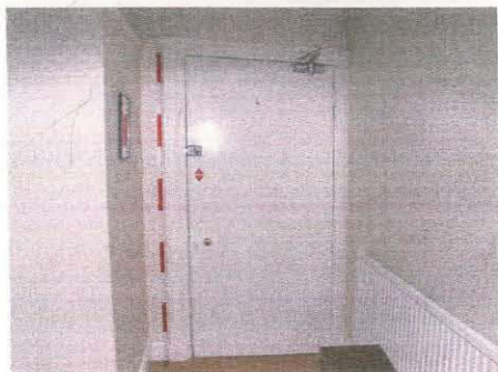
89. Detail of door (Room 40) showing moulded panel on the left jamb and possibly 19 th century rim-lock, taken from the west
