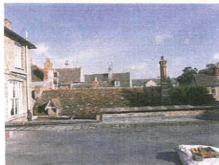
101. View over rooftops of Units 3, 2, 1 and 8, taken from the south (flat roof of Unit 12)
