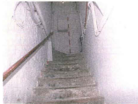
18. Stone stair to cellar of Unit 1 with blocked aperture at the top indicating an originally external wall, taken from the west
