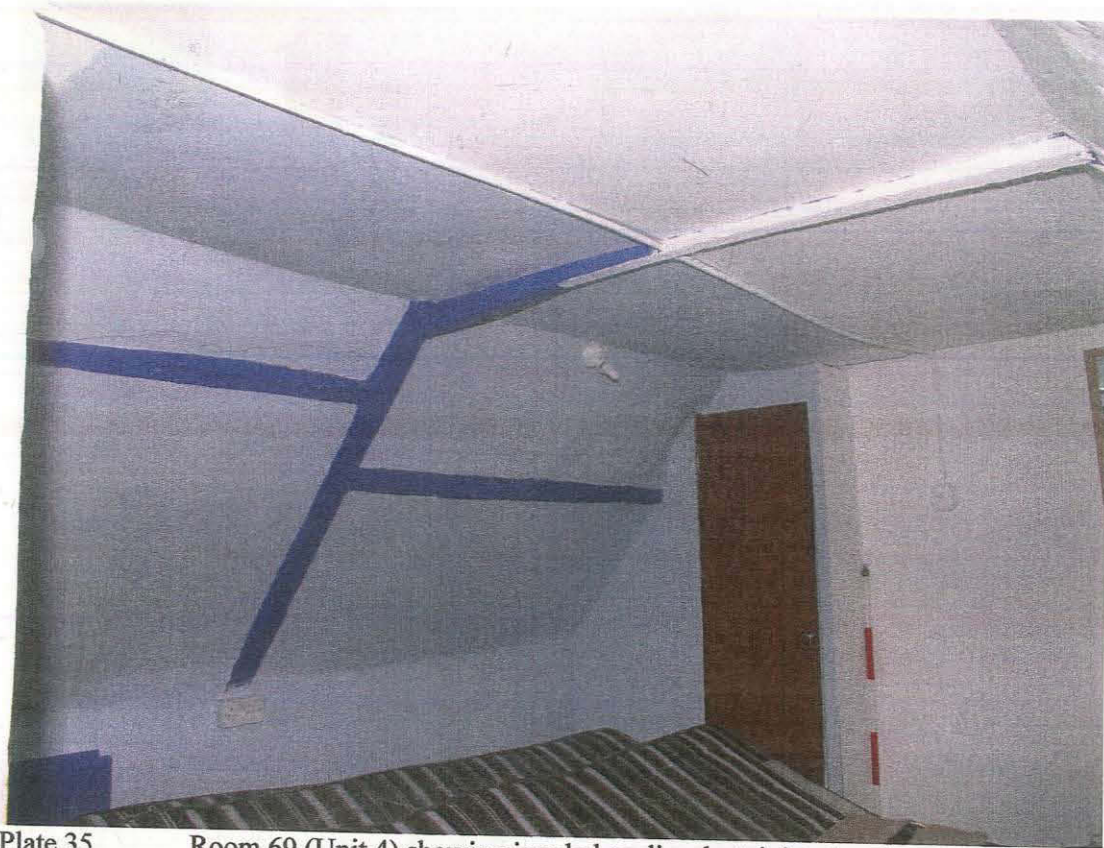
Plate 35 Room 69 (Unit 4) showing joggled purlins, butt-jointed to the rafters, taken from the north-west (143)
