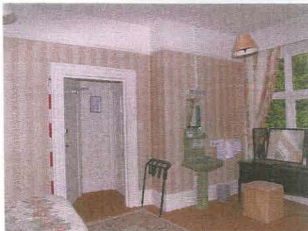
165. Room 61 showing original doorway and door to bathroom inserted at east end of the corridor, taken from the south-west
