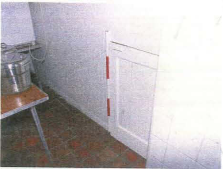
29. Understair cupboard in Unit 8; originally this would have been open to the stairs, taken from the south-east
