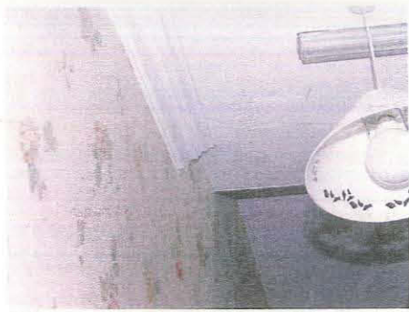
129. Break in ceiling and termination of cornice on the first floor landing of Unit 1, taken from the west
