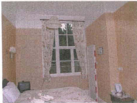
139. Room 46 (Unit 3) showing partition wall to north truncating the window, taken from the west
