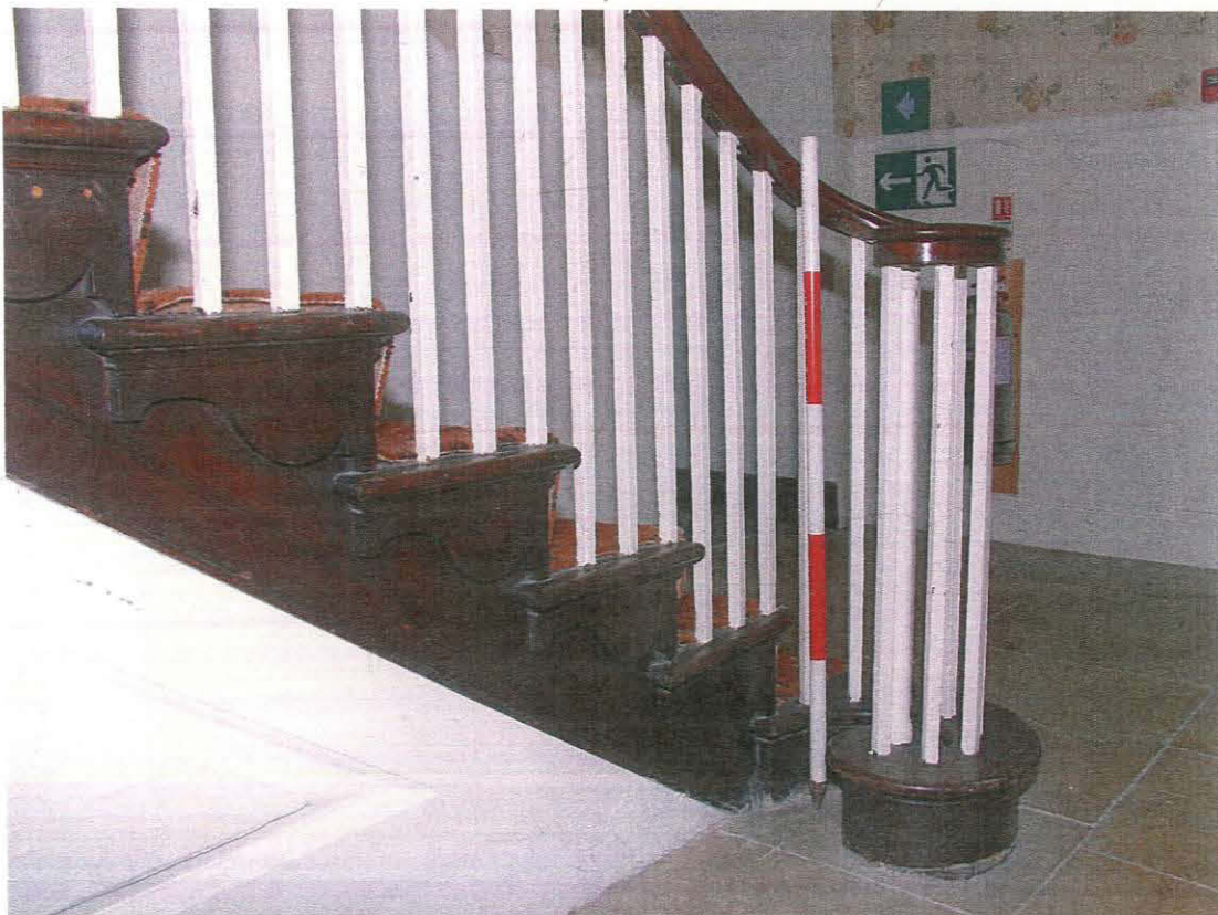
Plate 10 Bracket decoration on tread-ends of open string stair in hall of Unit 1, taken from the north-east (12)
