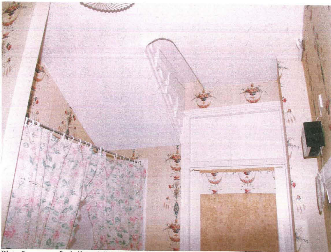
Plate 8 Stair line visible in the ceiling of Room 5 (Unit 1), showing the west wall inserted, taken from the east (16)
