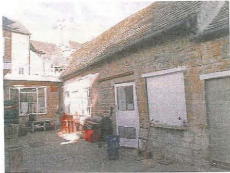
104. East elevation of Unit 9 and south elevation of Unit 8, taken from the south-east
