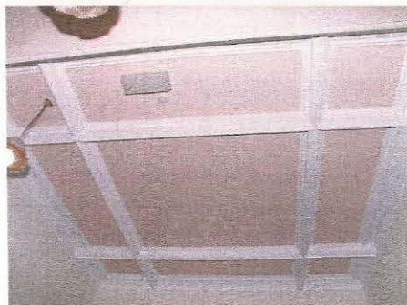
49. Detail of moulded joists in panelled ceiling of entrance lobby, taken from the south
