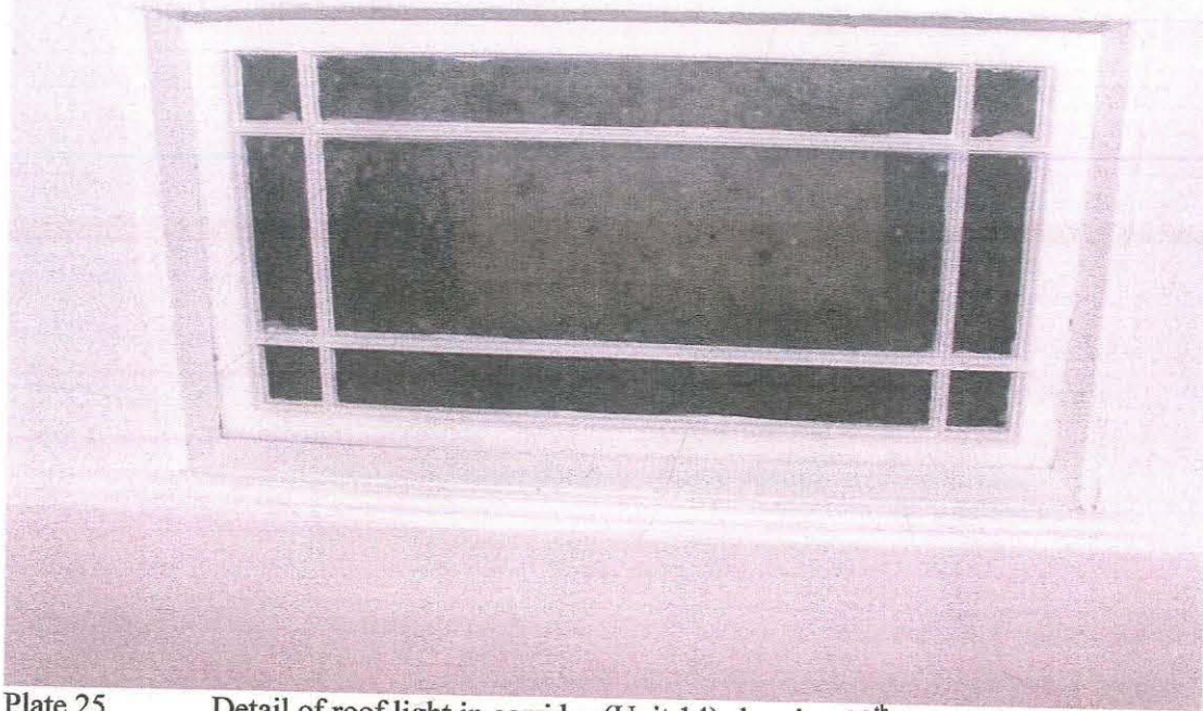
Plate 25 Detail of roof light in corridor (Unit 14) showing 19 th century etched glass, taken from the north (159)
