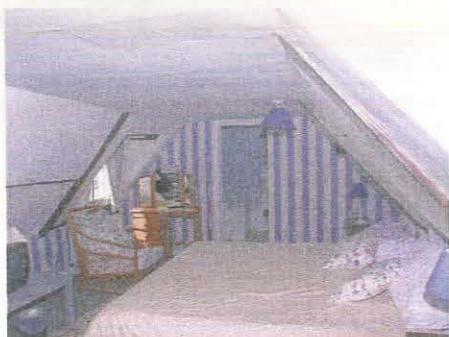
171. Room 63 (Unit 1) showing principal rafters with joggled butt purlins and dormer window, taken from the south-east
