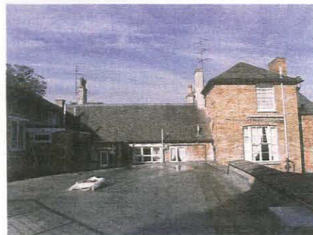
98. East elevation of Units 4 (left) and 3, taken from the east (flat roof of Unit 12)
