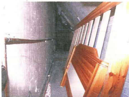
169. View into roof space (Unit 1) showing floor level change, taken from the west
