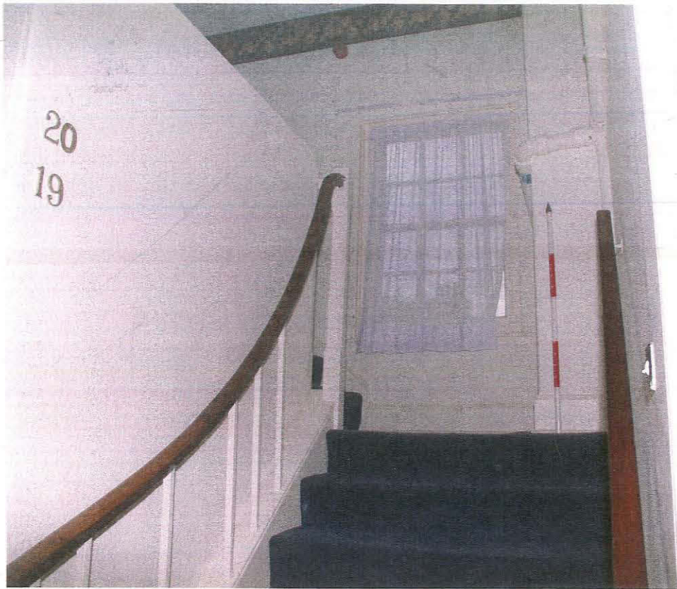
Plate 33 Shared stair of Units 2 and 3 between the first floor and second floor, taken from the south-west (135)
