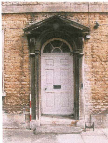
128. Detail of the central doorway in the west elevation of Unit 1, taken from the west
