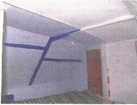
143. Room 69 (Unit 4) showing joggled purlins, butt-jointed to the rafters, taken from the north-west
