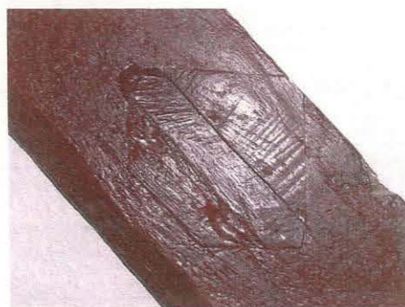
174. Detail of joint where purlin has been cut through in Room 64, taken from the south
