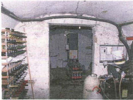
73. View from cellar Room 27 through to cellar Room 26 (Unit 4), taken from the south
