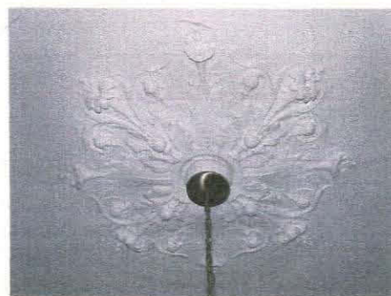
6. Detail of elaborate ceiling rosette enriched with leaves and lilies within Room 1, taken from the south
