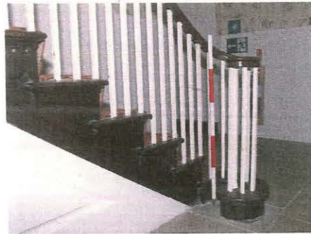
12. Bracket decoration on tread-ends of open string stair in hall of Unit 1, taken from the north-east
