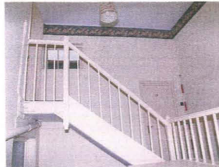
136. Shared stair of Units 2 and 3 between the first floor and second floor, taken from the south-east
