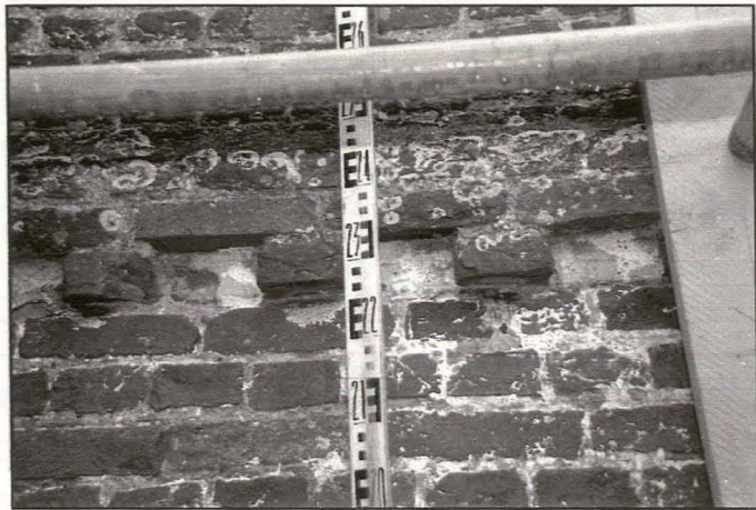
Plate 7: West Elevation showing denticulated stringcourse. Again, note the use of lime render infill between adjacent dentils complementing the treatment of the window detailing.
