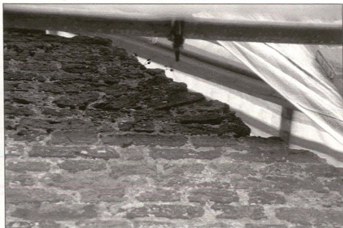
Plate 9: West Gable showing one of the fragments of 'Tumbling-in'. Sections also survive on the East Gable and indicate that the building originally had parapet gables.
