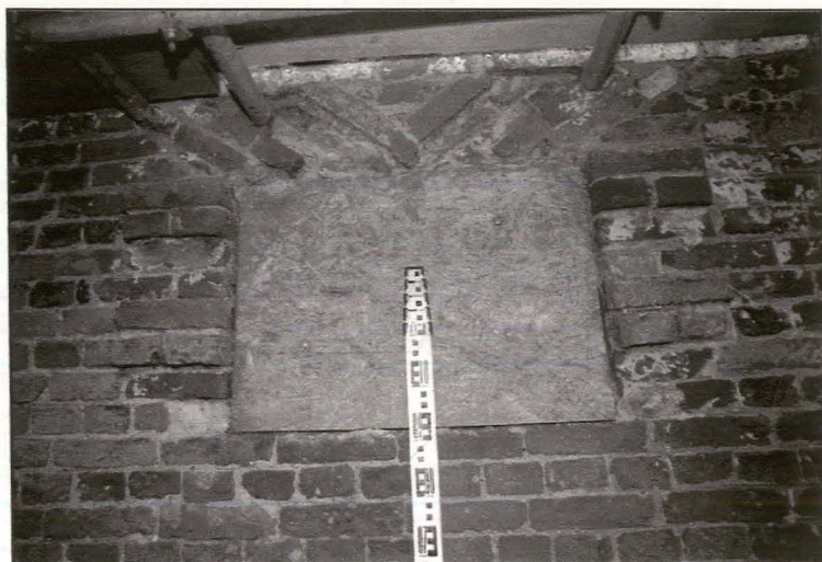
Plate 4: North Elevation, primary window of Unit A, showing the plain rustication to the jambs and the Dutch or French Arch that typifies the detailing of the original architectural design and characterises the building as belonging to the artisan mannerist tradition.
