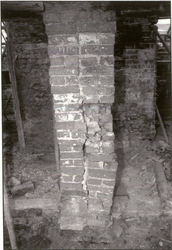
Plate 28: In contrast to the general quality of brickwork, which is generally fair to good, the central rusticated pier between the two front doors of the South Elevation is poor.
