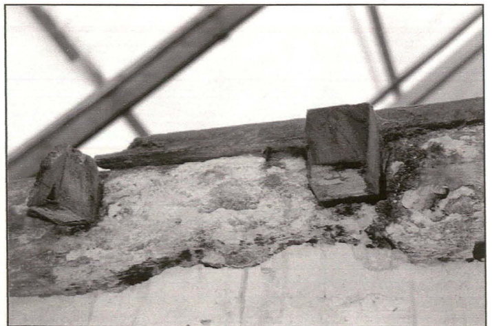
Plate 27: Unit B, this plate shows relict floor joists in oak still in situ . They are quartered and fit into sockets cut into the surviving tiebeam. The tiebeam is also in oak, boxed, and is finished with an ogee-stopped chamfer as per the fireplace beams.
