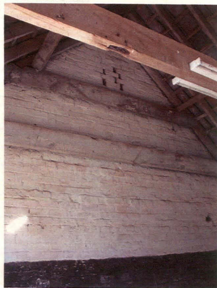
Plate 8 NW-SE Range, NW wall of 3 rd room from north showing ventilator holes, looking north
