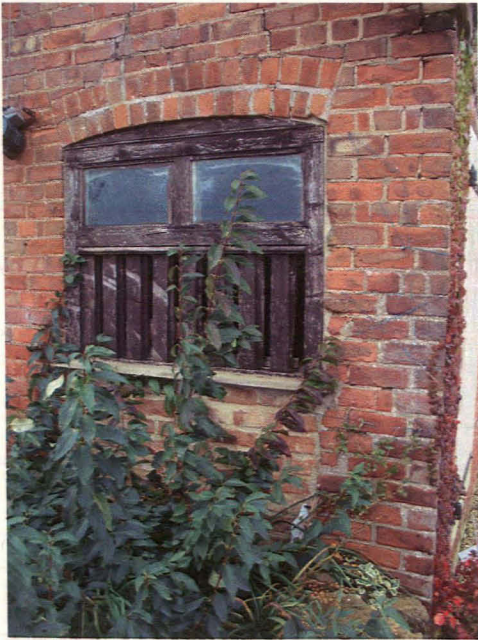
Plate 11 NW-SE Range, SE room, showing ventilator window in blocked door, looking west
