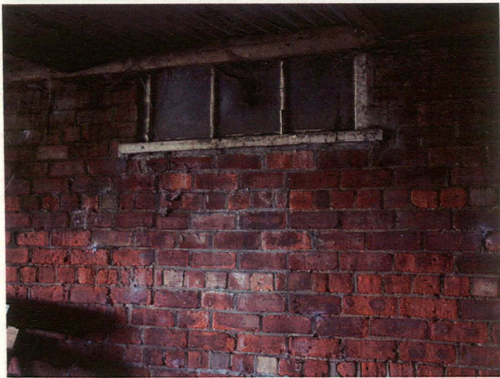
Plate 3 NW-SE Range, northwest external wall, showing straight joins of blocked window, looking southeast
