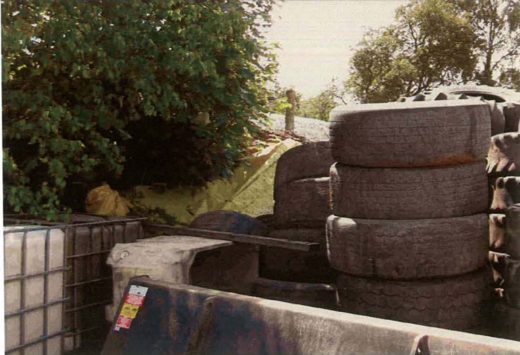
Plate 13 View toward extension (Room 3), showing chimney and roof, and stacked materials preventing access, looking west
