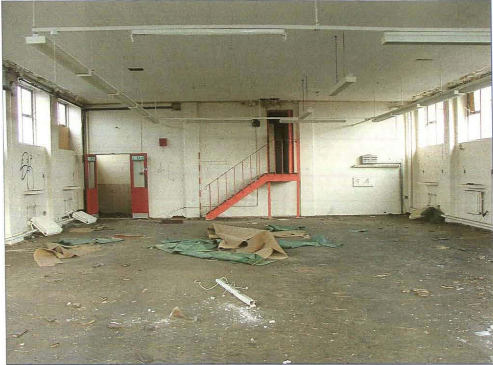
Plate 43. View looking north-east of the Operating Room showing metal stairs to rooms at second floor level (Scale = 2m)
