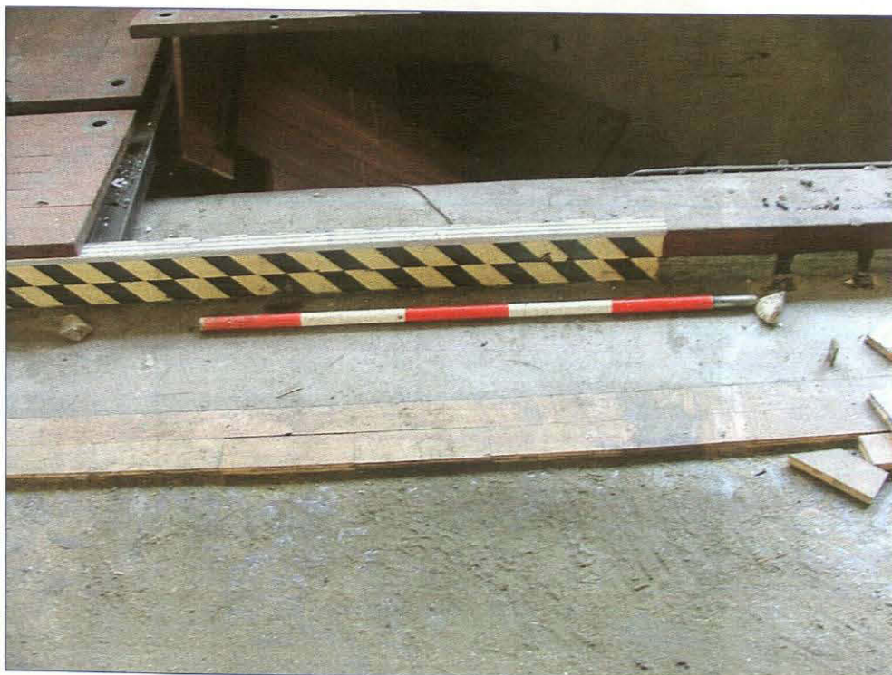
Plate 26. Surviving edges of a former parquet floor, ground floor large hall (Scale = 1m)
