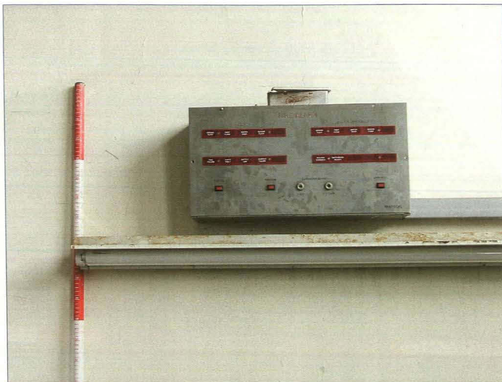
Plate 45. Detail of Fire Alarm System, Operating Room
