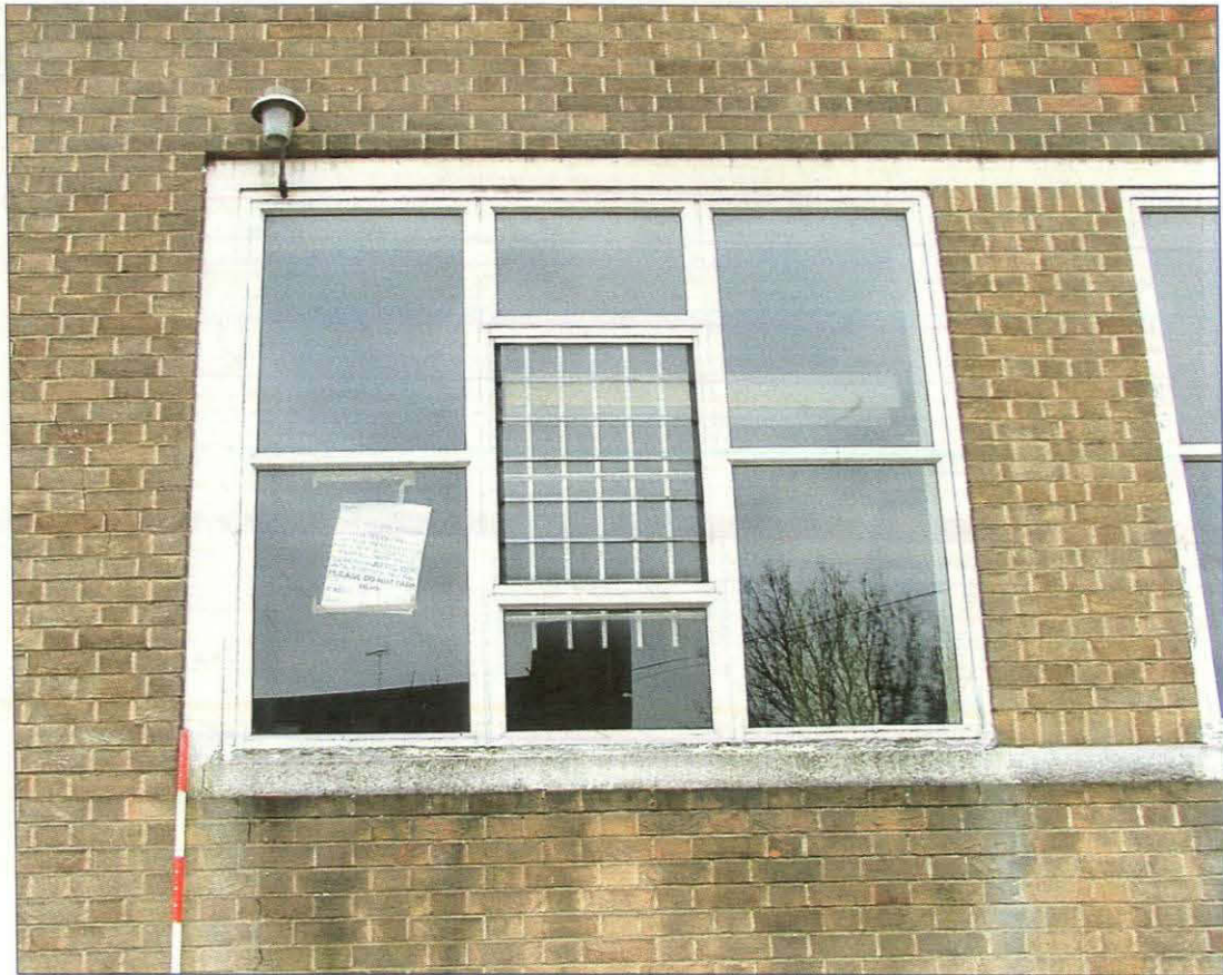
Plate 7. Detail of one of the windows in the single-storey extension, north-west elevation
