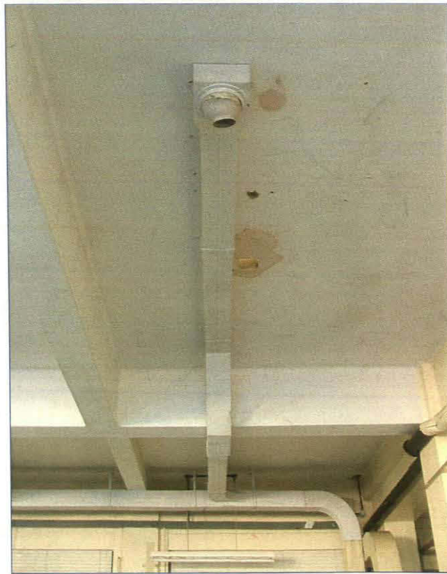
Plate 32. One of the lengths of ducting on the ceiling of the ground floor hall
