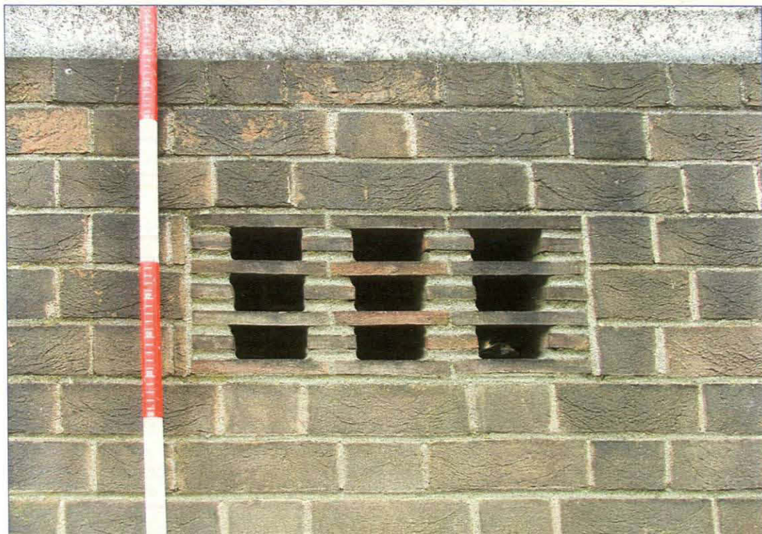
Plate 8. Detail of one of the ventilation holes, north-west elevation (each red and white section of the scale = 20cm)
