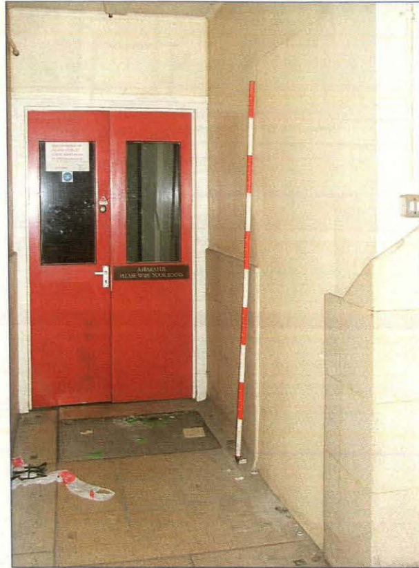
Plate 23. Former doorway to office as seen from the base of the stairs at ground floor level (Scale = 2m)
