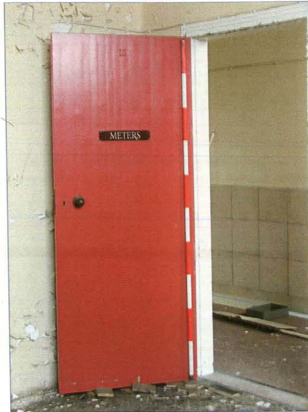
Plate 41. View of Meter Room door which displays the number '13' and the sign 'Meters' (Scale = 2m)
