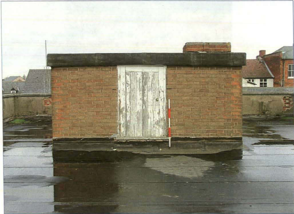
Plate 51. View looking north-west of small building on roof which houses the water tanks and access ladder (Scale = 1m)
