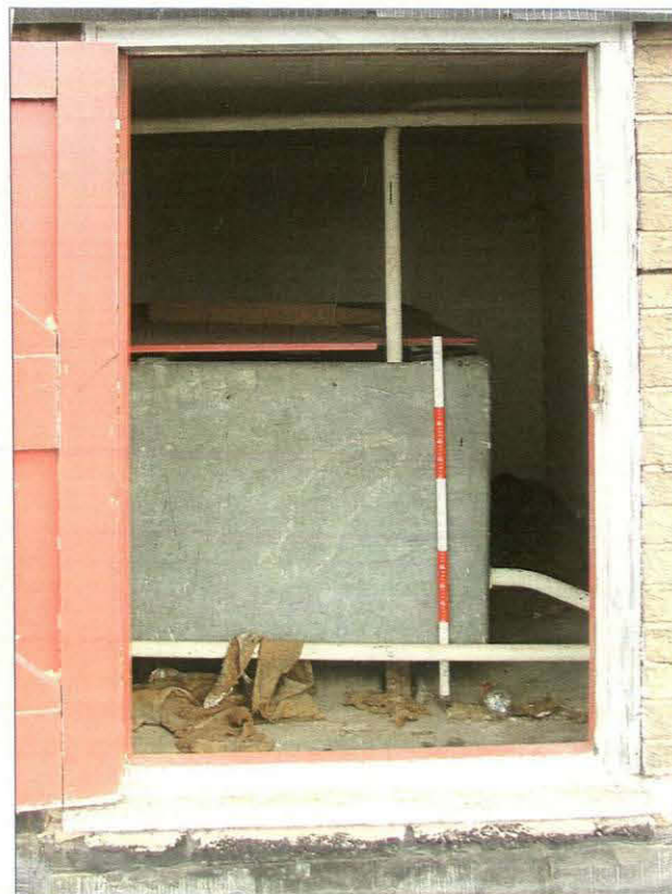
Plate 50. One of the two water tanks in the small building on the roof (Scale = 1m)
