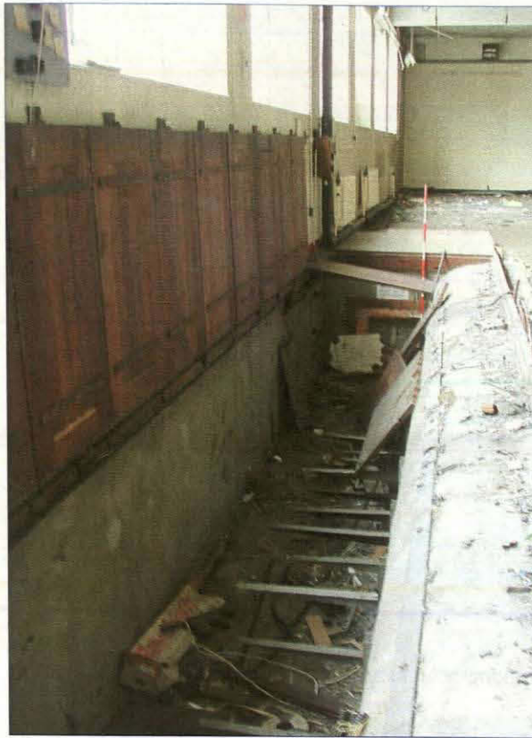
Plate 27. View looking north-east of the concrete pit in ground floor hall with wooden hatches (Scale = 2m)
