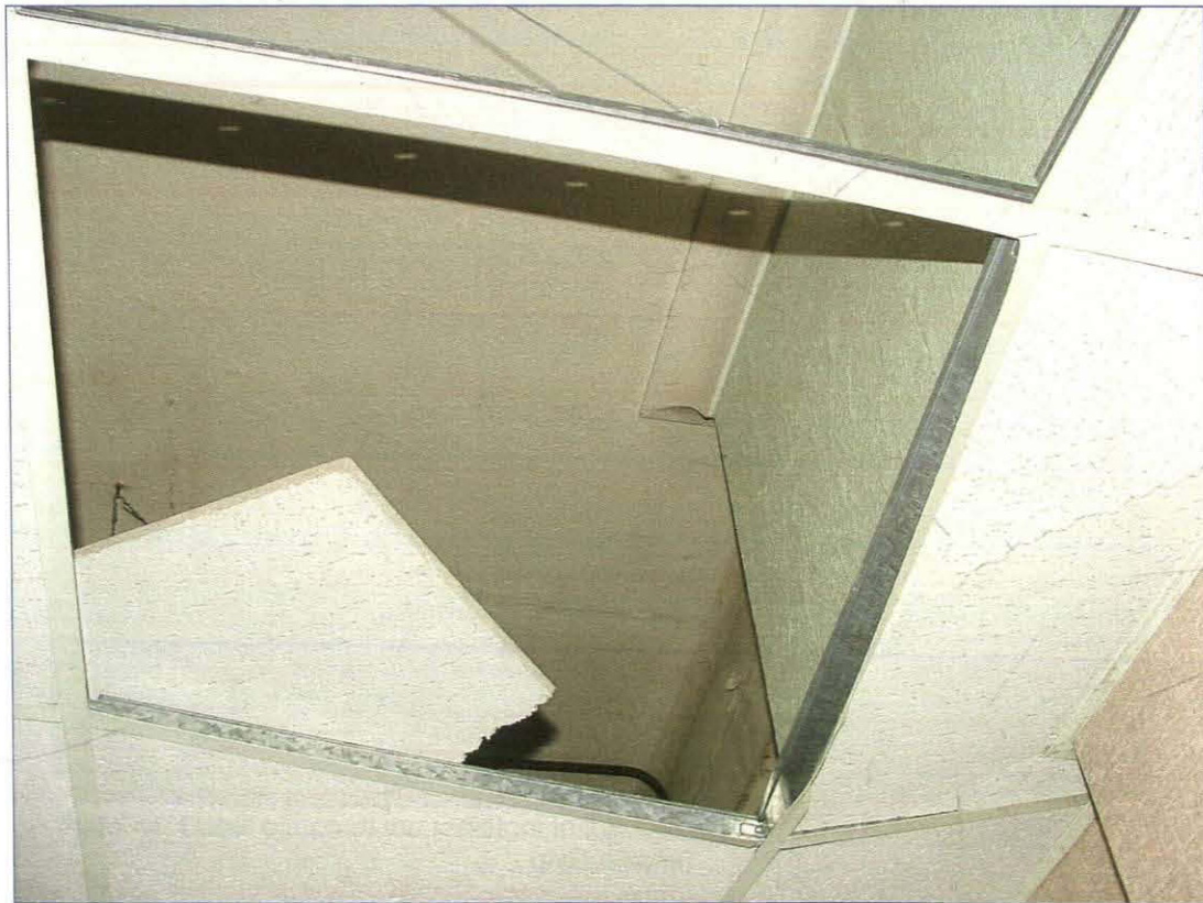
Plate 48. Second floor office, showing coving at top of the wall partially hidden by the suspended ceiling
