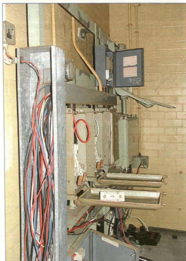
Plate 16. View of the remaining electrical equipment in the Electrical Intake Room, ground floor
