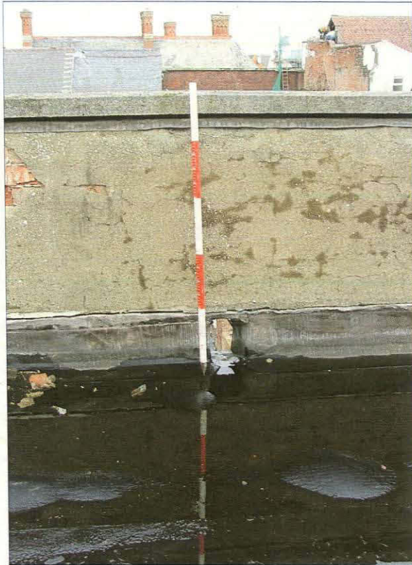
Plate 55. Detail of one of the drainage holes at the base of the parapet which allows water to drain into the hoppers
