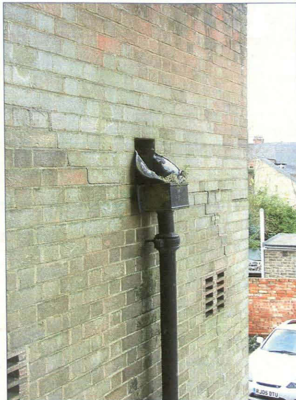
Plate 9. Detail of the rain water hopper, north-east facing elevation of single-store extension, as seen from within the first floor office
