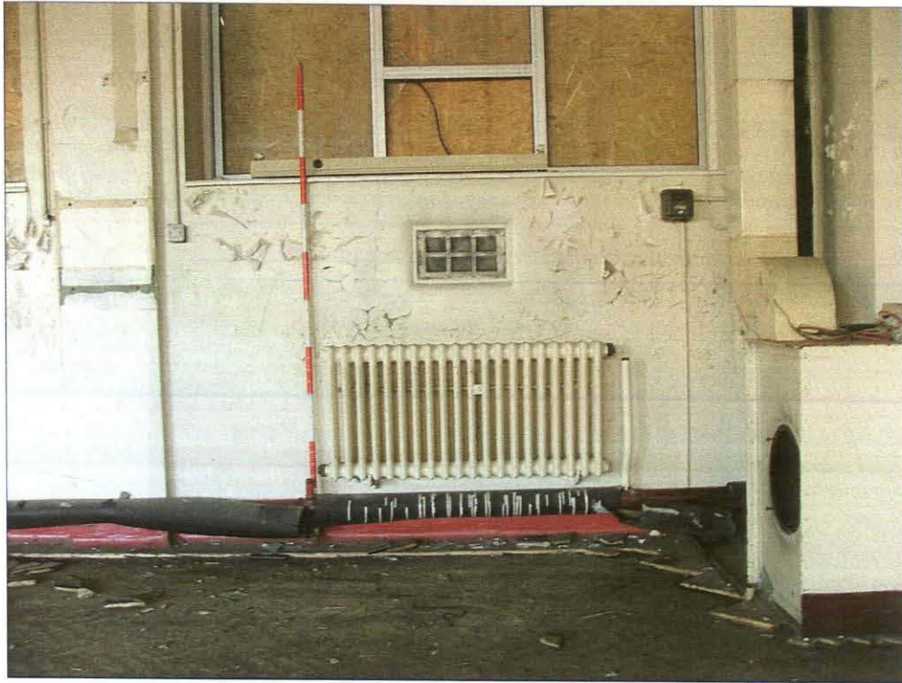
Plate 29. Detail of one of the radiators, ground floor hall (Scale = 2m)
