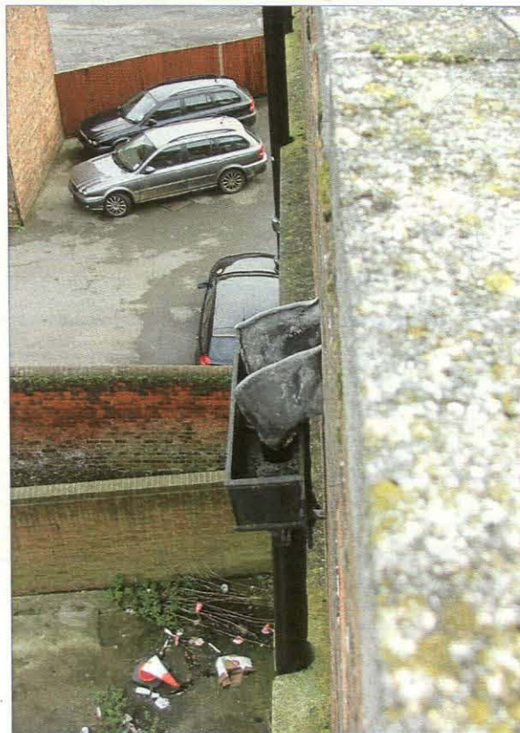
Plate 56. Detail of one of the rainwater hoppers as seen from the roof
