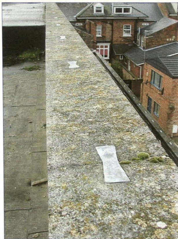
Plate 54. Detail of lead ties between the concrete capping stones of the parapet
