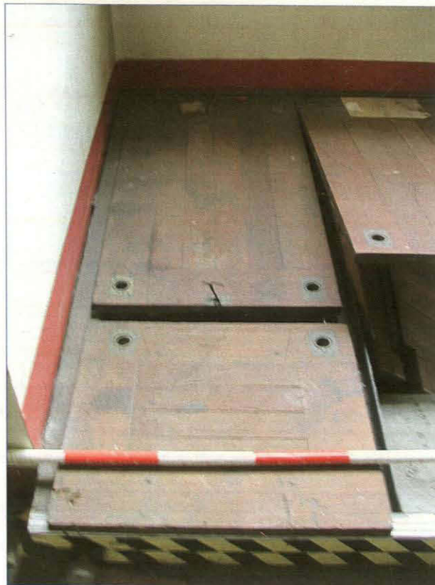
Plate 28. Detail of some of the wooden hatches over the pit, ground floor (Scale is in 20cm graduations)
