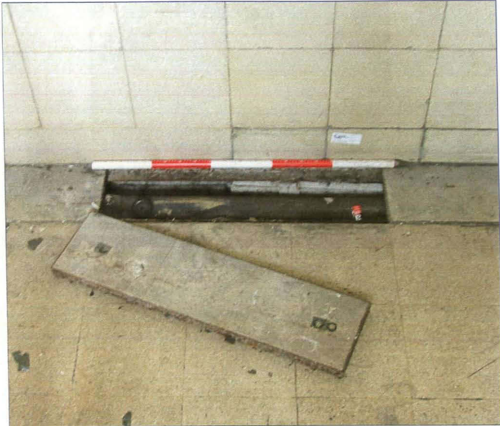
Plate 19. Heating pipe located beneath the floor of the entrance hall (Scale = 1m)
