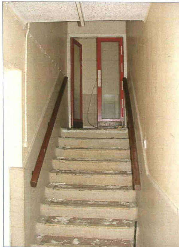
Plate 40. View from first floor landing looking towards stairs and doors to Operating Room (Scale = 2m)
