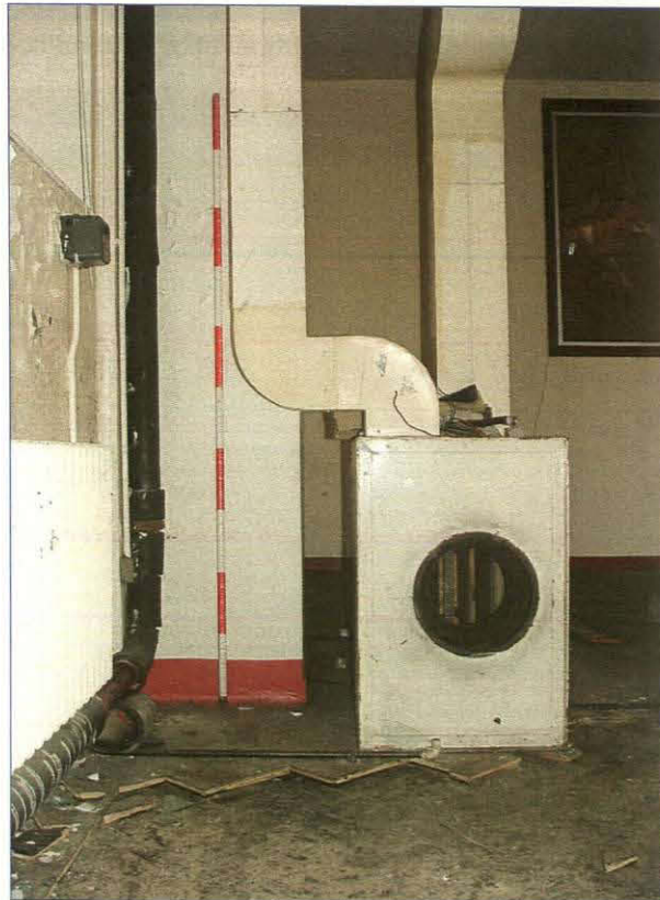
Plate 30. Fan unit casing, ground floor hall (Scale = 2m)
