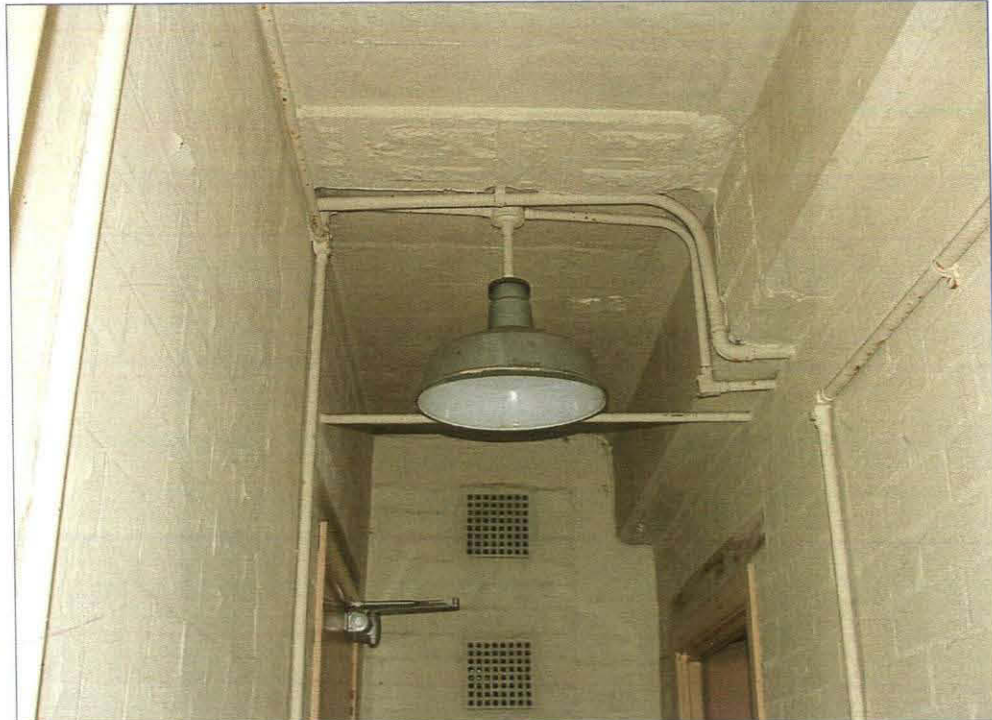
Plate 20. Light shade in ground floor corridor to the Tank Room and Boiler Room
