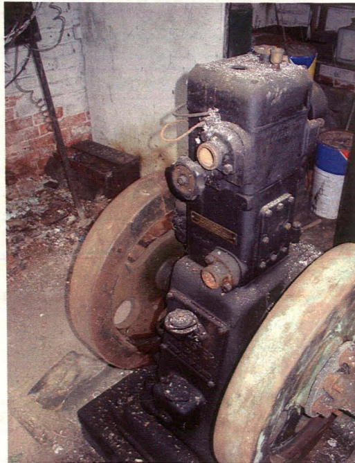
Plate 9 Front section of large generator, looking NE
