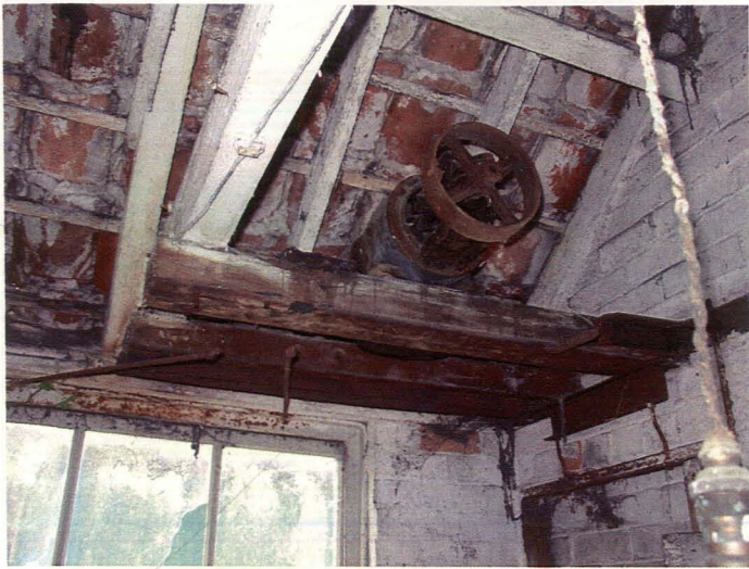
Plate 12 Overhead smaller generator supported by girders
