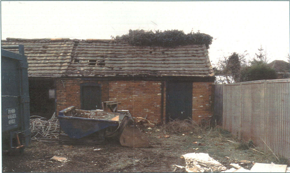
Pl. 3: Exterior view of Rooms A & B, looking west. Note area of rebuilding around the door of Room B. Note also that the roof tiles have been removed (compare to fig. 1)
