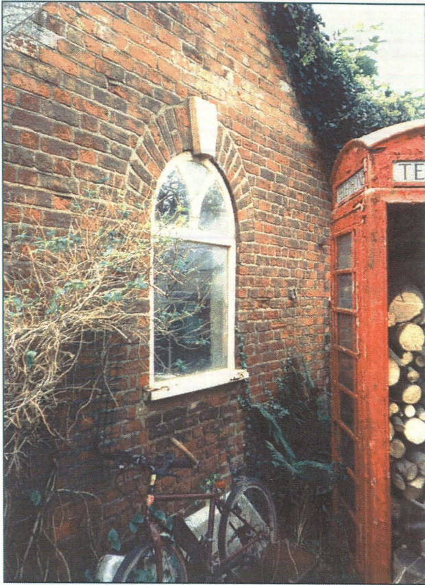
Pl. 5: External view of decorative window in north wall of Room A, looking south-west (J. Bonnor, LCC).
