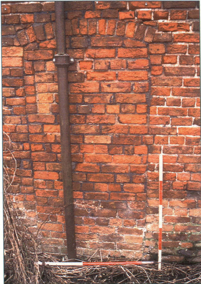
Pl. 17: Detailed view of blocked doorway in exterior of Room E. Looking east.
