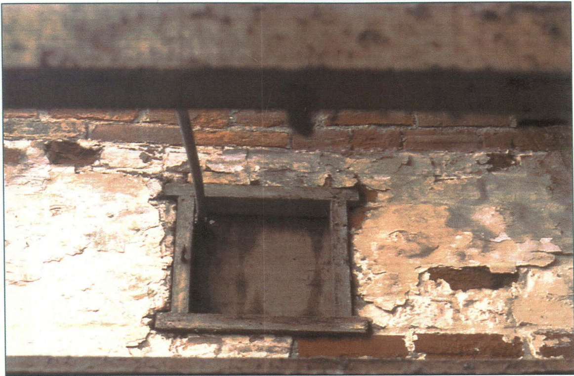
Pl. 11: Possible ventilation hatch in upper south wall of Room D. Looking south
