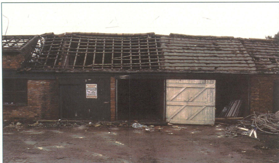
Pl. 8: Exterior view of Rooms C & D, looking west. Note the modern window and brickwork of Room E to the left of the shot
