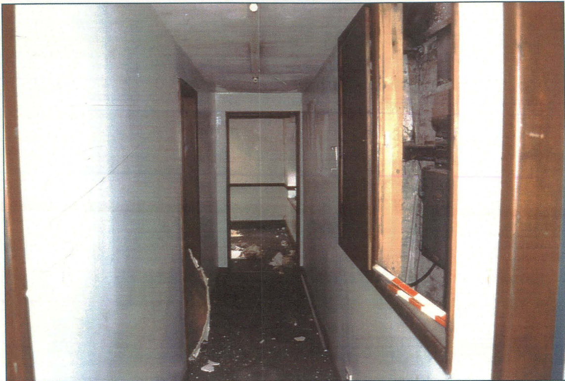
Pl. 13: Corridor to Room H, looking west. The original wall is visible in the fuse box to the right.
