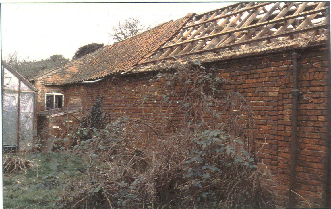
Pl. 16: View along western exterior wall, looking north. Note the hatch in Room D, and the blocked doorway at the extreme right of the shot
