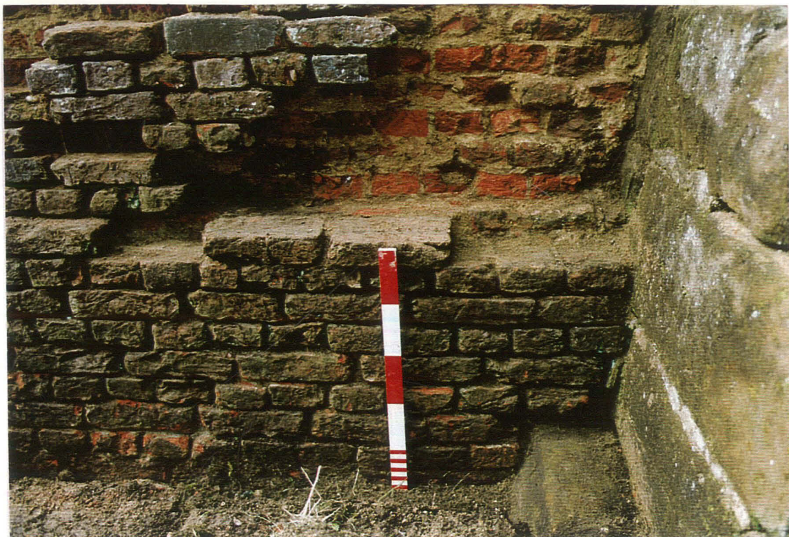
Pl. 6 Elevation A. Detail at west end showing brickwork built over stonework of Elevation B. Scale 0.50m
