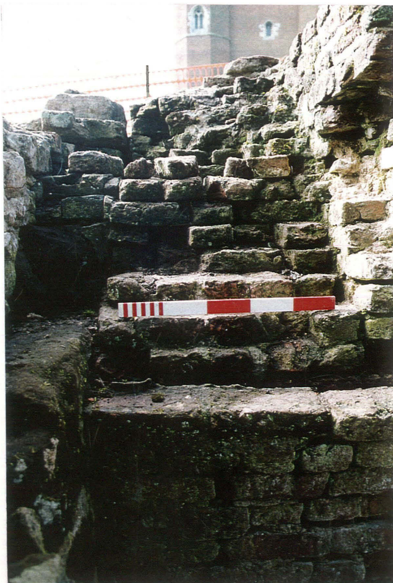
Pl. 21 Elevation I at junction with Elevation H, after cleaning, showing straight joint. Scale 0.50m
