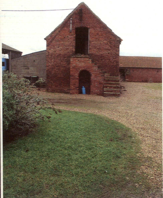
Plate 6 - West facing elevation of the north range showing staircase to first floor
