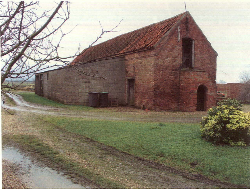
Plate 7 - View showing the concrete lean to on the north side of the north range
