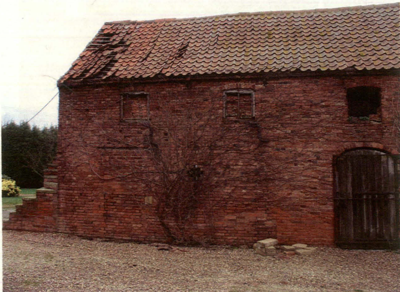
Plate 3 - South elevation of the north range showing blocked door and window openings for the first floor
