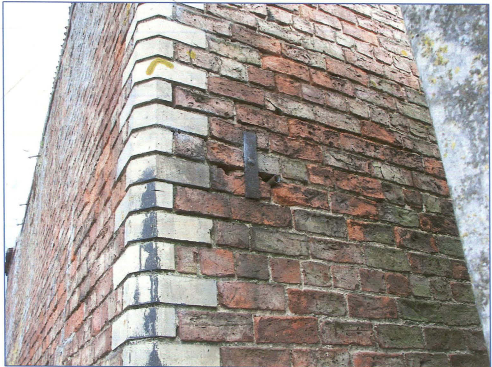
Plate 5 (Shot 24): Shot taken looking north-east of the south-west corner of the barn showing the polychrome detailing using single cant bricks in a gault fabric at the corners of the barn. To the right is a simple tie plate.
