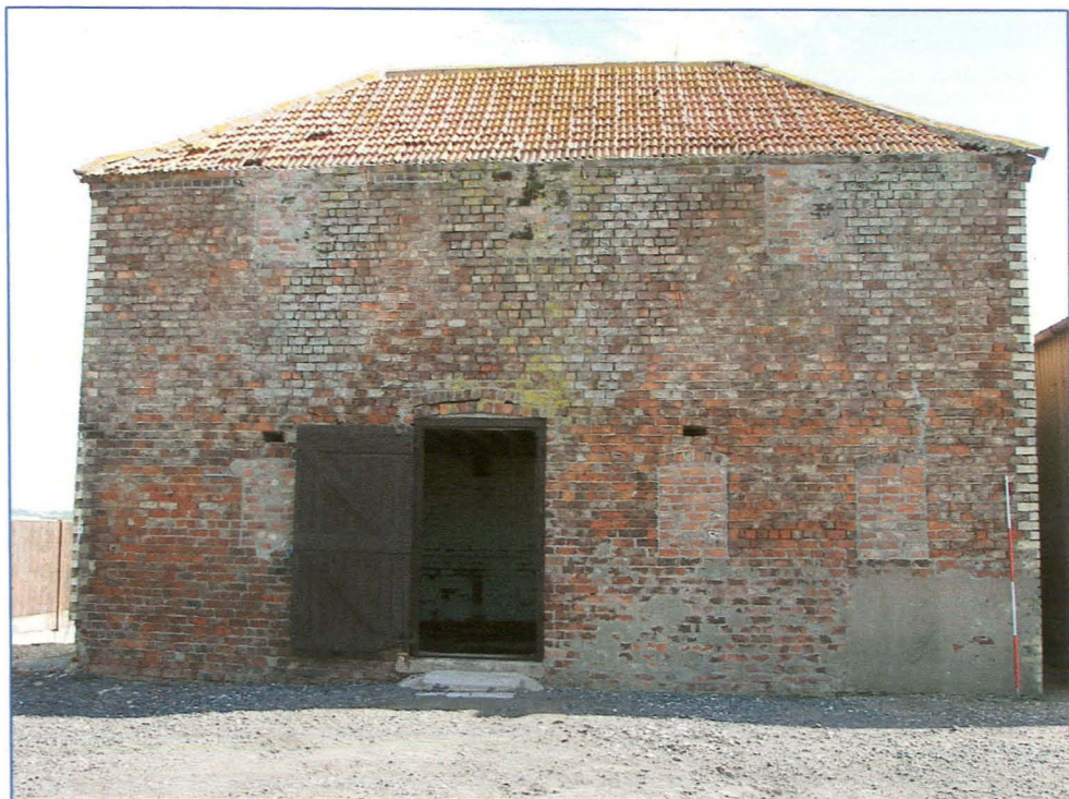
Plate 2 (Shot 5): The south-west facing elevation showing the blocked in windows on the ground and first floors. Looking north-east.
