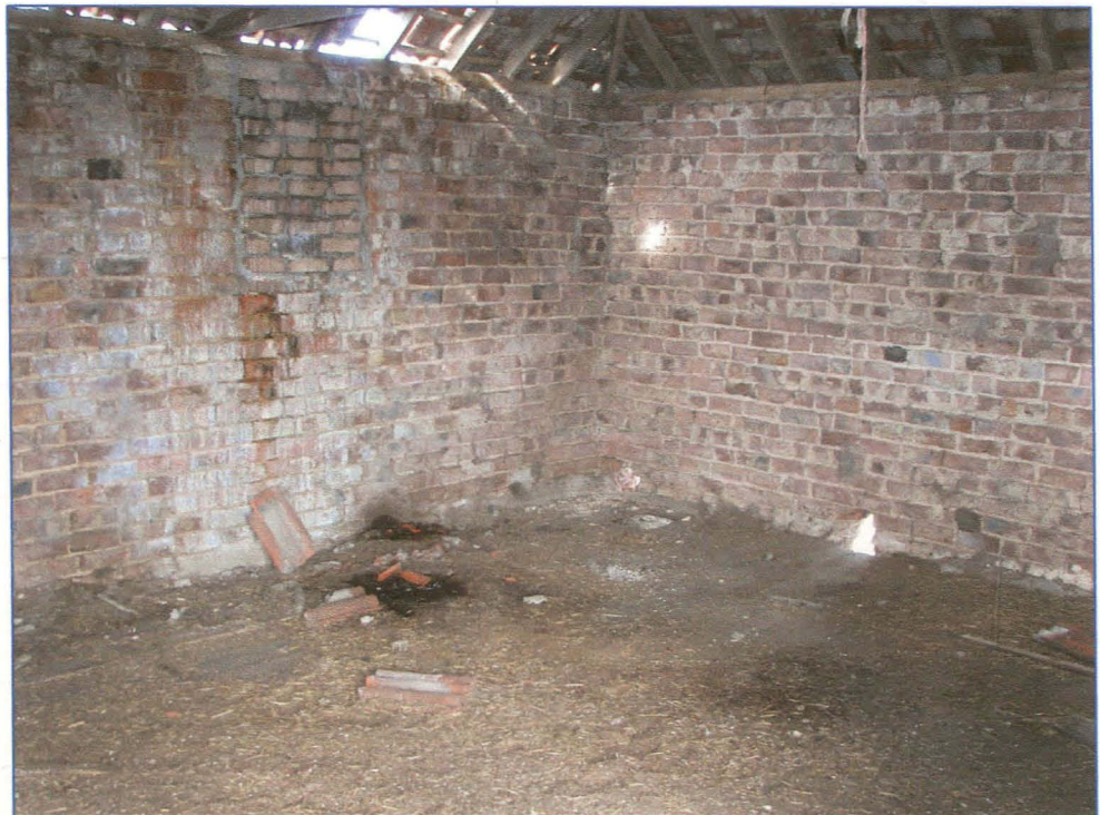
Plate 12 (Shot 28): Internal shot of the empty first floor looking south-west. Note the blocked window in the south-west wall
