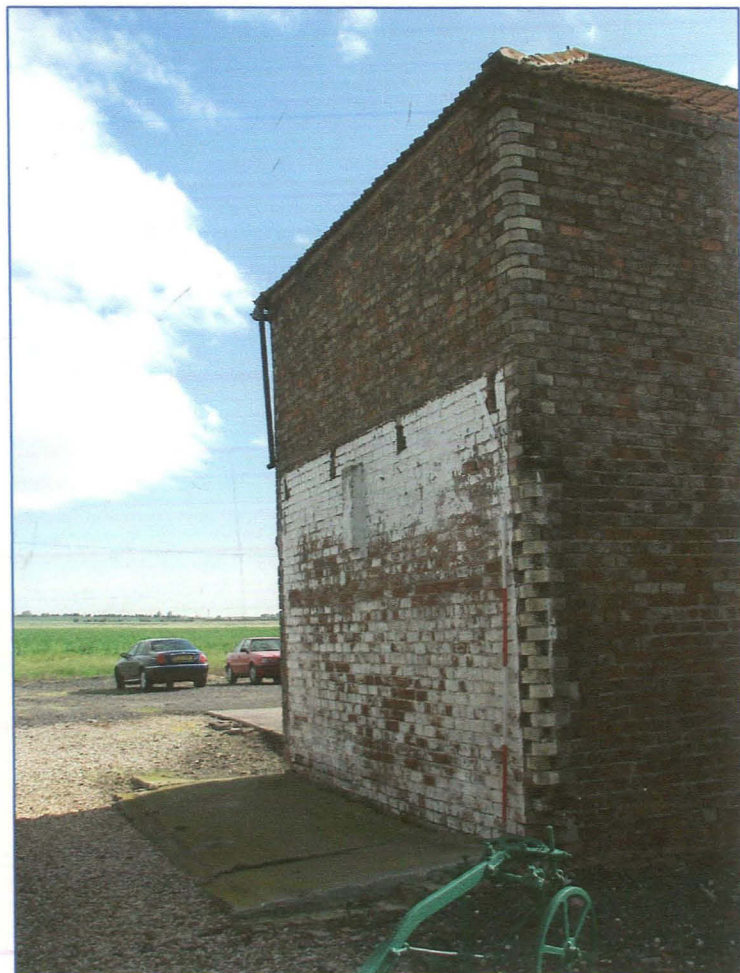
Plate 4 (Shot 9): The north-west facing elevation, looking north, showing the scarring from the recently demolished outbuilding and the surviving concrete floor.
