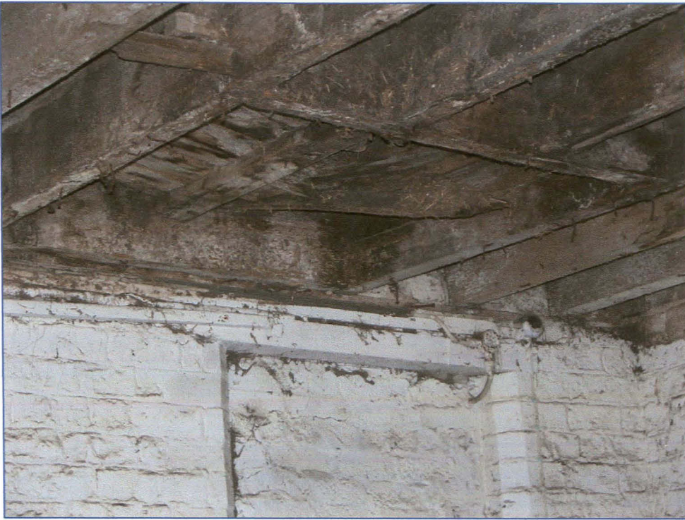
Plate 11 (Shot 31): A blocked opening in the first floor joists that formerly housed an internal staircase. The opening is located in the north-east corner of the barn over the blocked external doorway, the shot was taken looking north-east.
