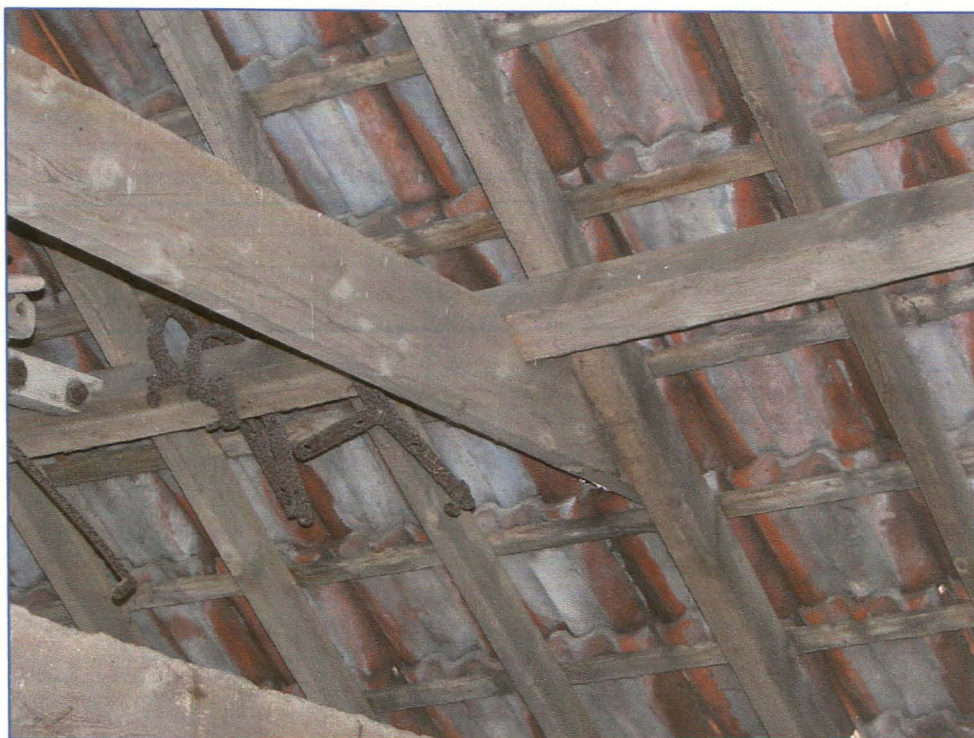
Plate 13 (Shot 30): Detail of the clasped purlin construction of the roof timbers, viewed looking south.
